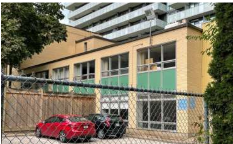
56. View of the west elevation of the 1959 east wing addition facing the courtyard and parking lot which are separated by a wood fence. (HP, 2021)
