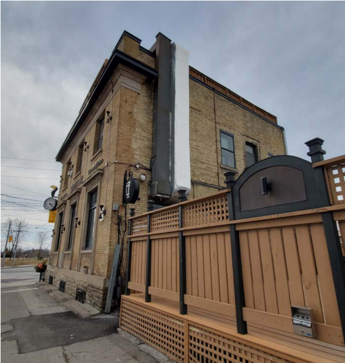
Figure 15. Detail of the corner quoining in the rear (north) elevation of 1702 Queen Street East (Heritage Planning, 2022)
