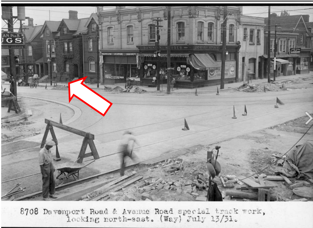
8708 Davenport Road & Avenue Road special track work, locking north-east. (Way) July 13/31. 7. 1931 archival photo looking northeast from the intersection of Avenue Road and Davenport, and showing the collection of four heritage properties at 177-183 Avenue Road built by the Woodley families. (City of Toronto Archives)
