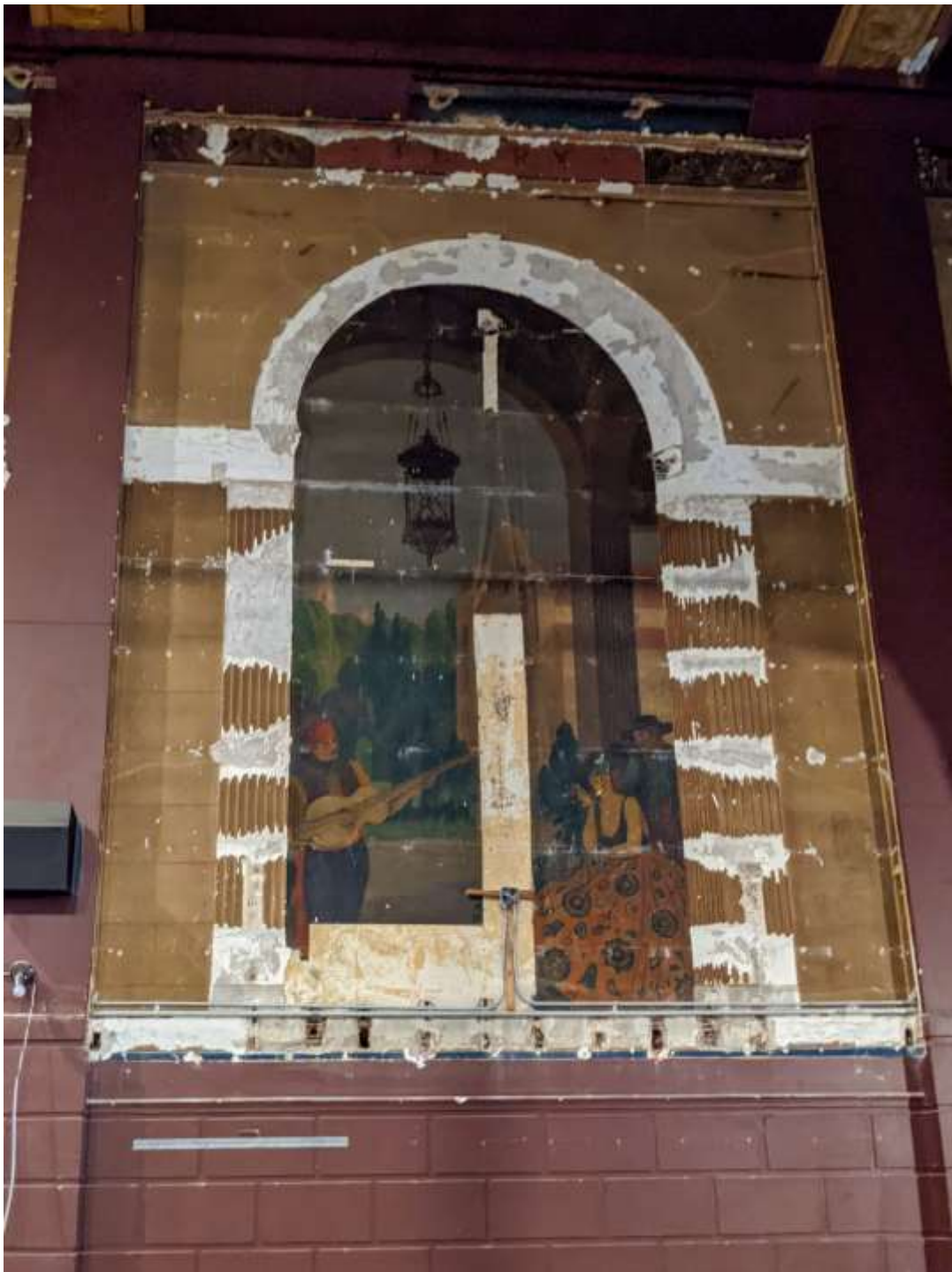
Figure 34. This image shows what remains of the north wall mural (one of two "friezes of Carmen, the Spanish dancer") and above, the inscription appearing to read "Terry" (a possible reference to actress Dame Ellen Terry). Much of the plasterwork on the auditorium walls has suffered damage and/or is missing as a result of previous renovations. (Heritage Planning, 2022).
