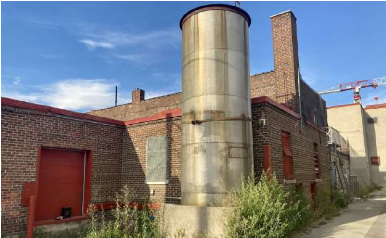
Figure 34: Southwest corner of the subject property, showing the c.1956 addition and 1960 steel tank, with the oldest (1920-1921) structure visible beyond, 2022. (Heritage Planning)
