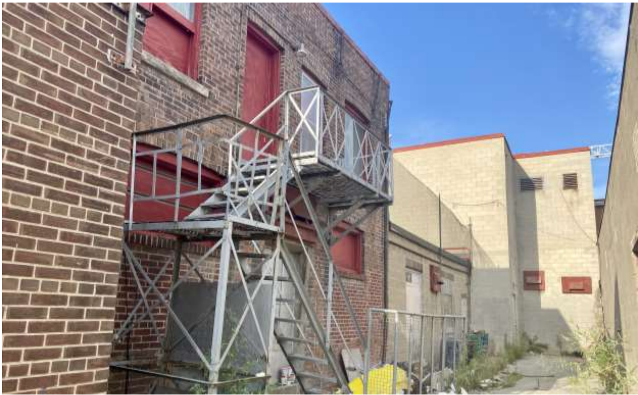
Figure 35: Northeastward view of the rear of the subject property, with the oldest (1920-1921) structure visible at left, 2022. (Heritage Planning)
