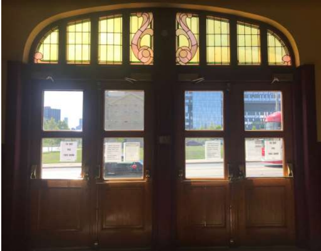
Image 27. Interior of the main entrance, looking out (west) at the former Don Jail site (Heritage Planning, 2022)
