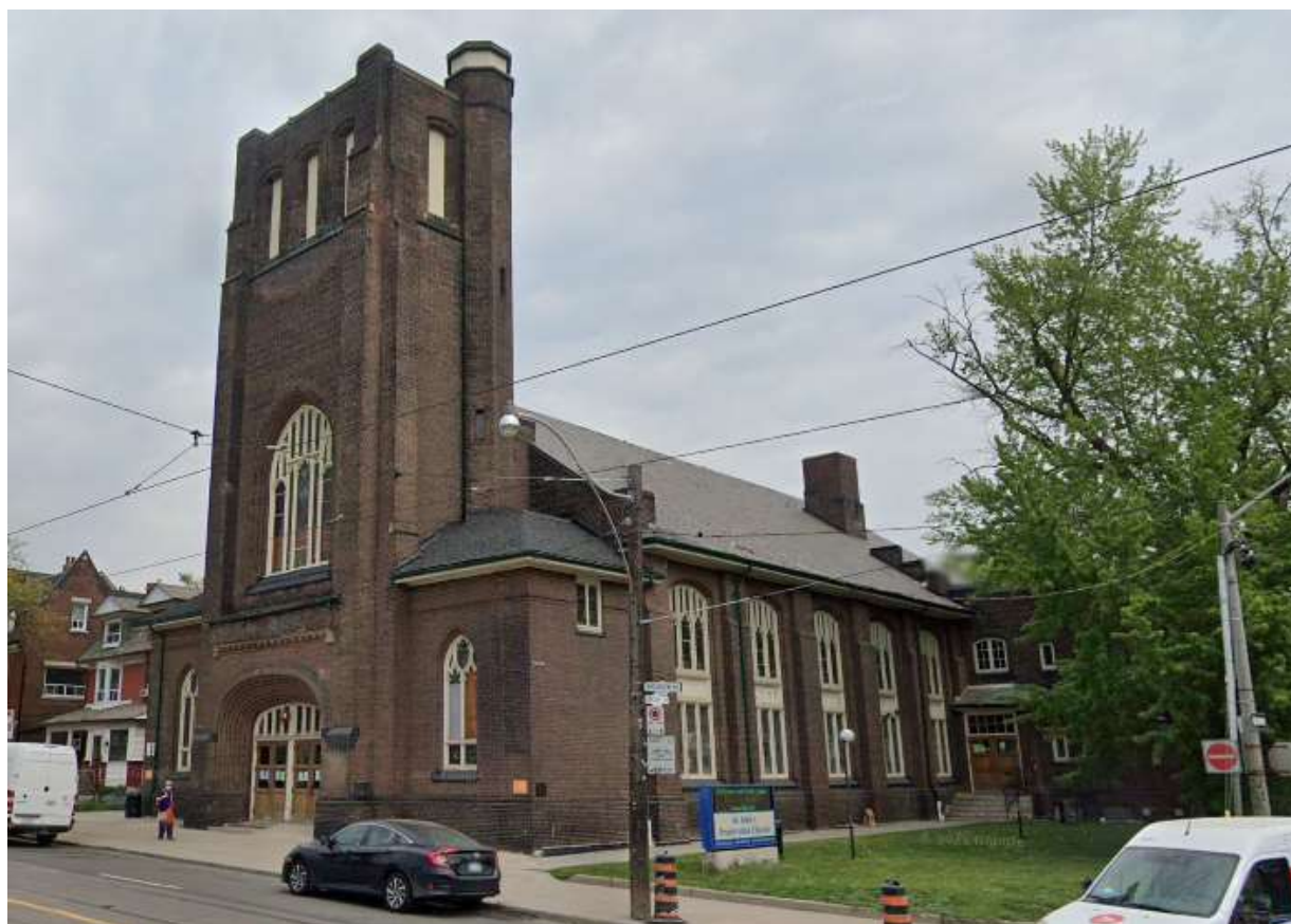
Current image showing the principal (west) and south elevations of St. John's Presbyterian Church.
