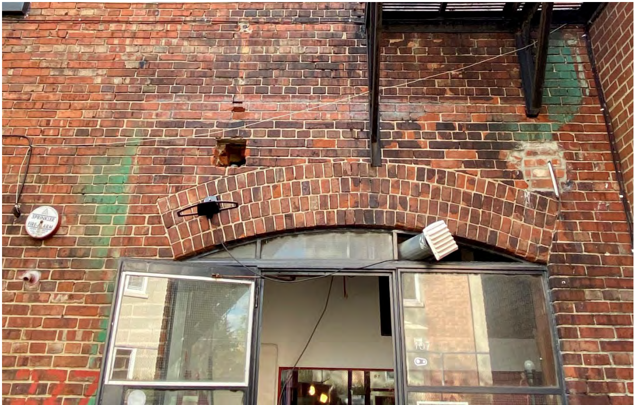
Figure 38: Upper level of the east elevation of an addition to the subject property, dating to c.1939, showing a brick row-lock arch. (Heritage Planning, 2021.)
