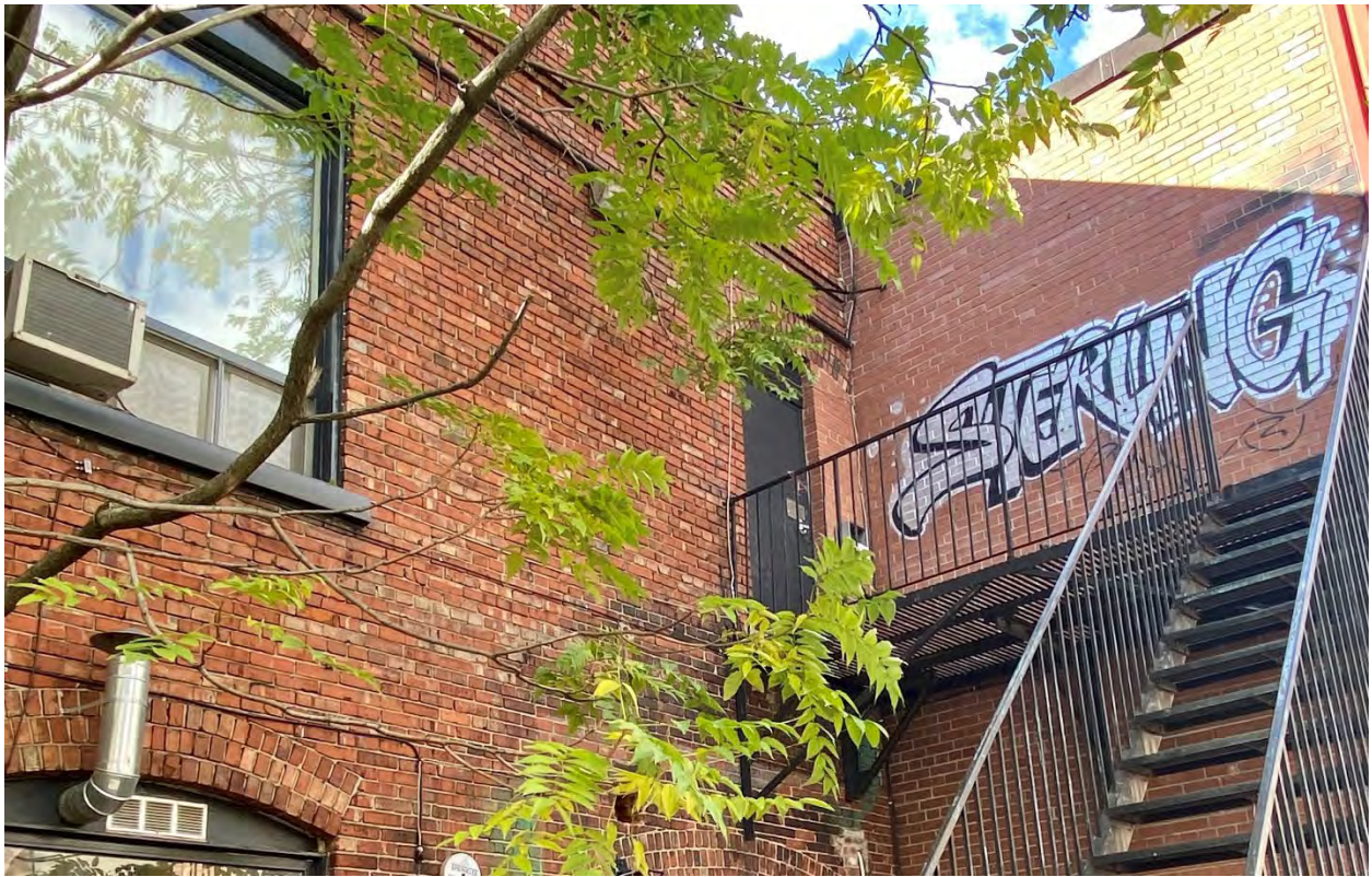
Figure 37: Upper level of the east elevation of an addition to the subject property, dating to c.1939, integrated to the north with a later addition (dating to c.1954-1965). (Heritage Planning, 2021.)
