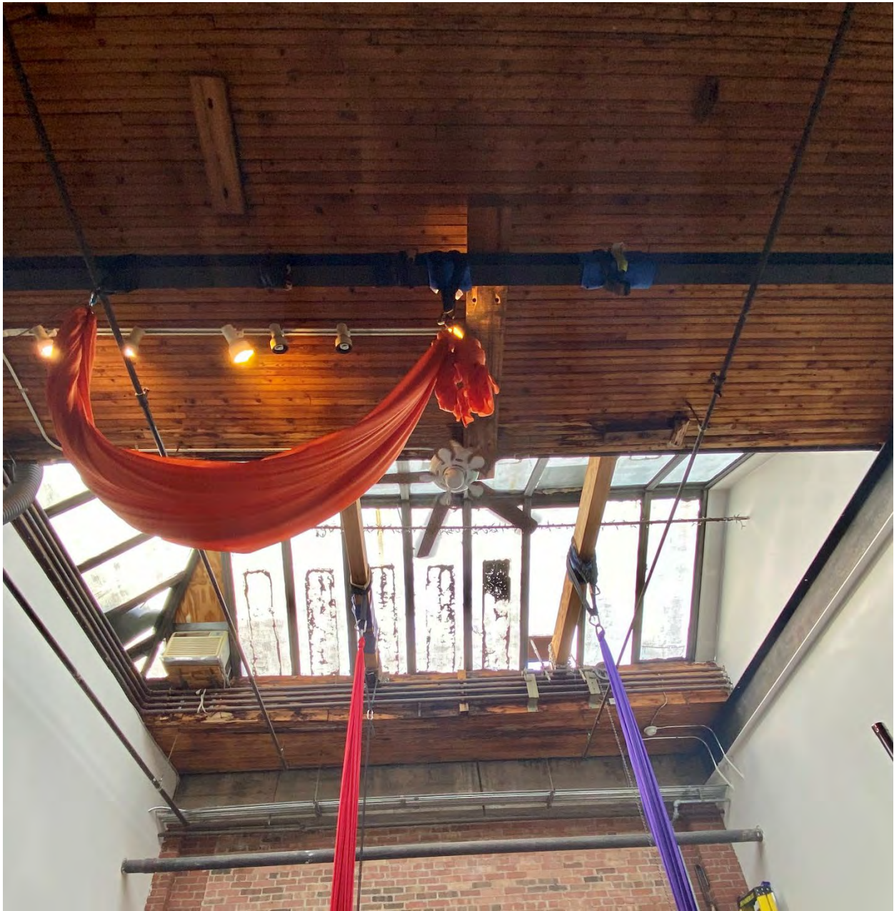
Figure 2: Interior of a unit within the southern portion of the subject property, showing high ceiling, skylight, and exposed beam currently used for rigging acrobatic equipment. (Heritage Planning, 2021)
