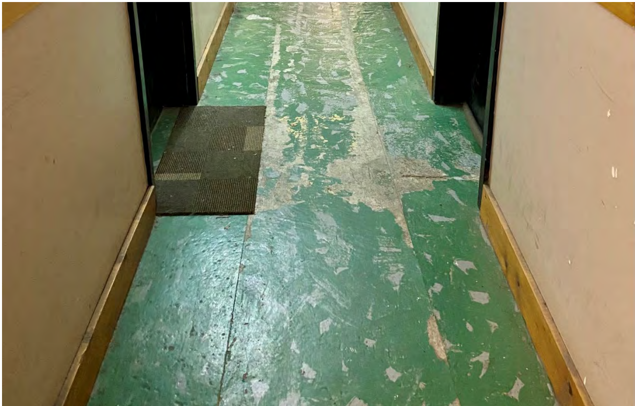
Figure 31: Interior corridor within the subject property's oldest portion, with original rail spurs appearing as two parallel lines along the floor. (Heritage Planning, 2021.)
