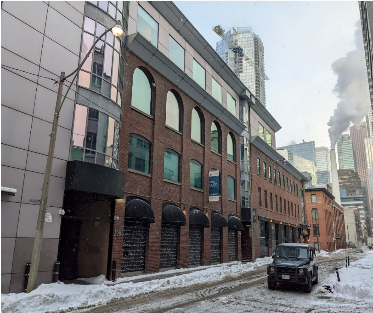
Figure 27. Detail of the side (south) elevation, illustrating the 1902 building (right) and the 1906 addition (left) with the fourth-storey addition that was re clad in the late-20 th century (Heritage Planning, 2022)
