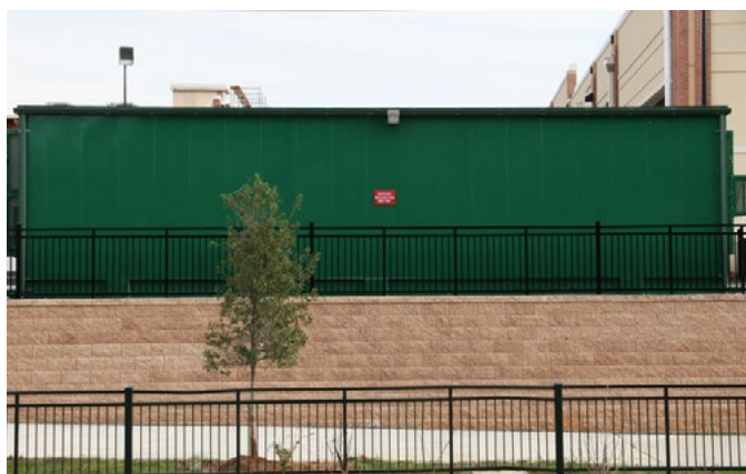
Figure 18: Substation prior to artistic treatment (Photo Credit: Leigh Brinkley, City of Charlotte)
