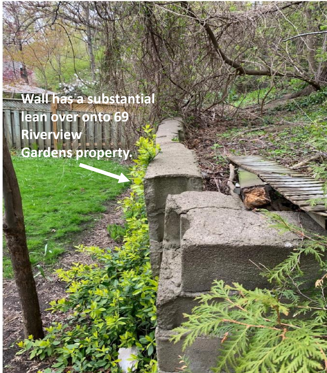
Figure 1. View showing wall leaning.
