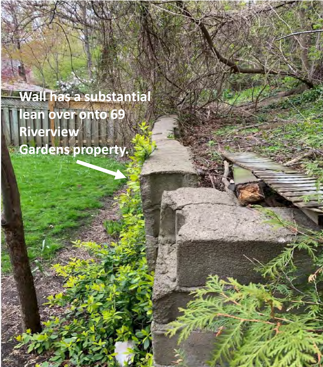
Figure 1. View showing wall leaning.
