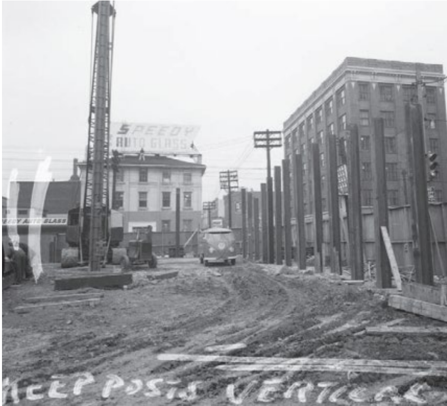
Image 17. 1957 image of the property looking west from University Avenue during construction (Panda Associates).
