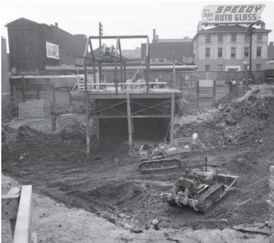
Image 18. 1958 image of the property looking west from University Avenue during construction (Panda Associates).
