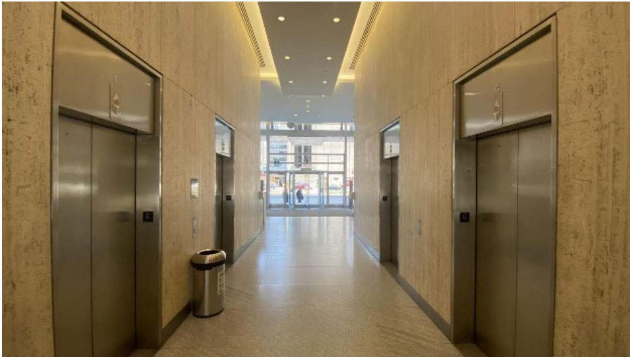
Image 43. Current photo looking east across the elevator lobby to the University Avenue entrance and showing the travertine wall panelling, granite floors, stainless steel elevator doors and surrounds, and drop ceiling panel with recessed pot lighting. (ERA, 2022)
