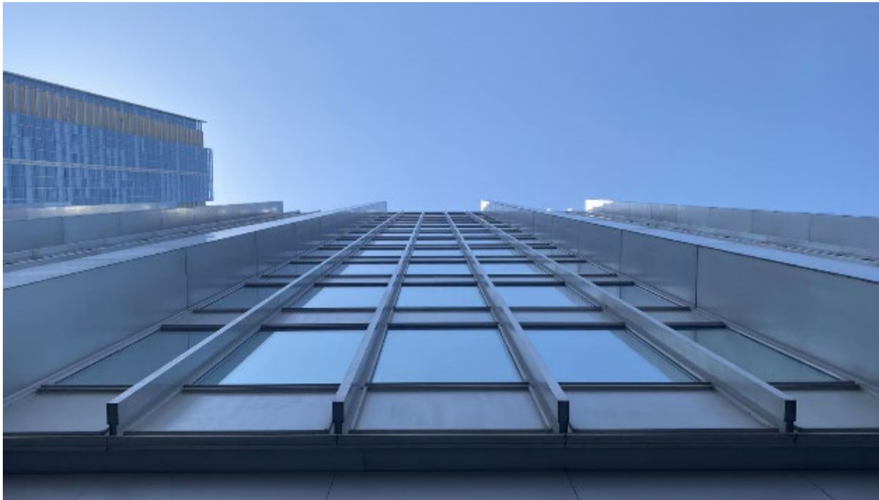
Image 37. Current photo looking up and showing the aluminum-clad "fins" (at centre) flanked by larger perimeter columns found on all four storeys of the building exterior and creating a strong sense of verticality. (ERA, 2022)
