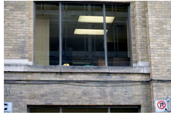
63. Many of the horizontal joints at window sills require repointing and sealing. PGA
