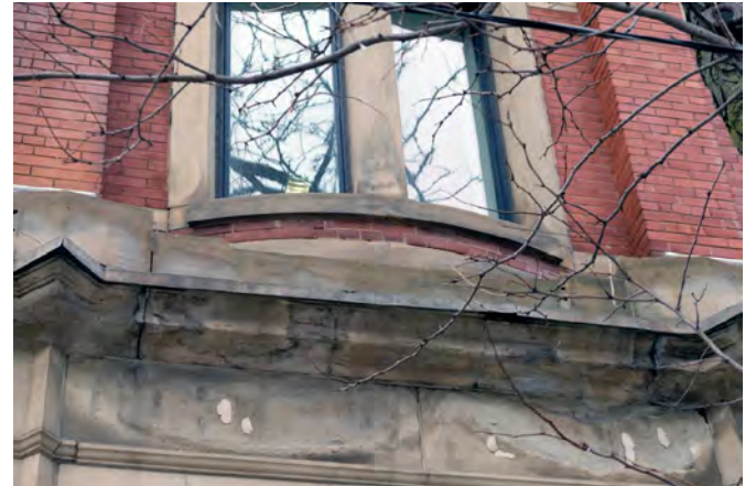
71. Detail view of stonework above the main entrance and below a shallow oriel window in the west bay of the front elevation. Staining and some stone erosion indicate leaks at horizontal joints above. Flashing has been added and should be repaired as required. PGA
