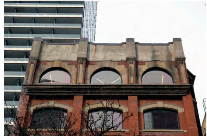
70. Detail view of parapet above the 6th floor. This area has been cement parged in the area where a large entablature and projecting cornice was formerly located. A metal cornice will be restored in this location to closely match the original as seen in historic photos. . PGA
