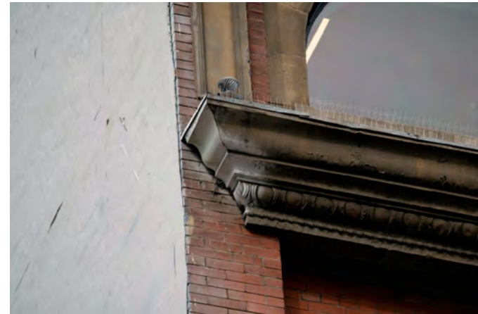
73. Detail of metal secondary cornice at 6th floor level. Note paint overspray. PGA
