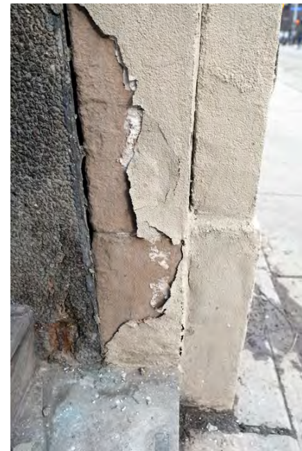
64. Detail at storefront pier 218 King W. Note peeling surface coating near grade. This may require removal and stone repair or consolidation. PGA
