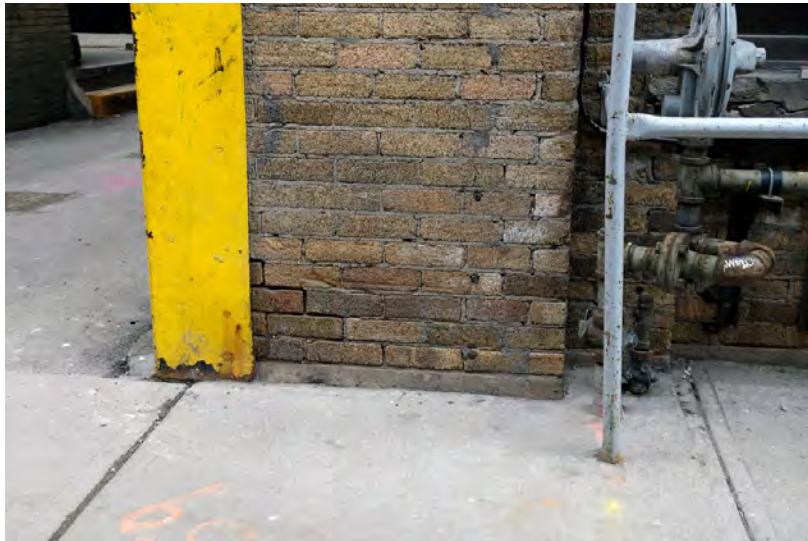
59. Detail at NE corner north side of open joints in brick near grade. PGA
