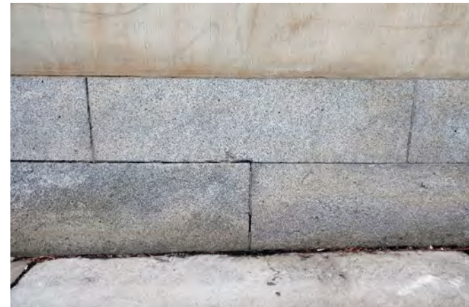
52. View of open joints in granite base along Simcoe St. PGA
