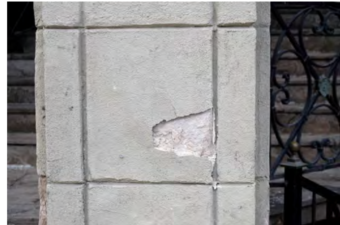
65. Detail at storefront pier 218 King W. The surface coating has been pushed off the dusting sandstone beneath. Generally the coating remains adhered, but in the long run may need removal so the stone can be refinished and possibly consolidated. PGA
