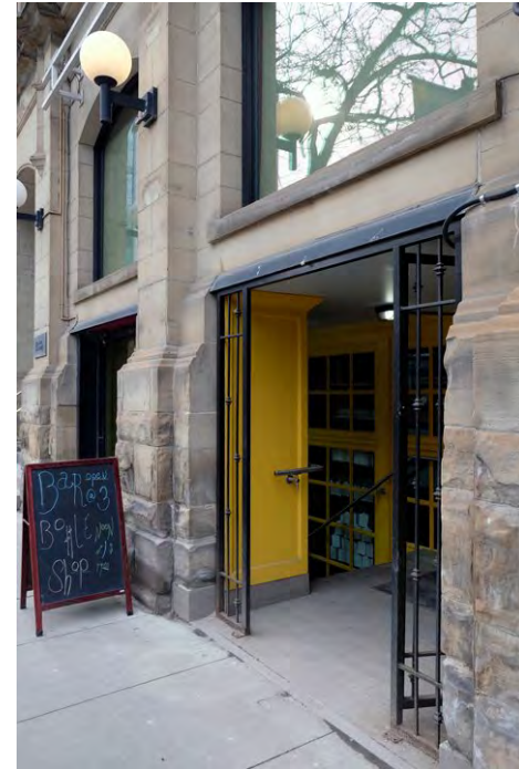
74. View of entrance to basement in an altered window opening at the east bay ground floor. The window opening should be restored with a new sill and possibly lintel. Note staining of stone from rising damp and de-icing salts. All open joints should be repointed. PGA
