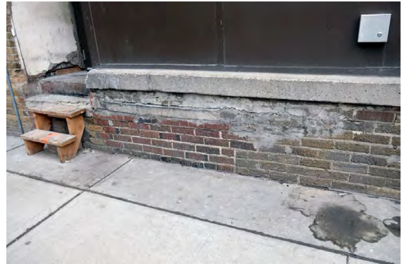
60. Detail at delivery "dock" all of these sills require reconstruction or repair. Closed openings will receive new windows. PGA
