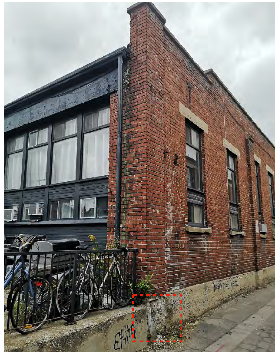
Corner of the west (left) and south(right) elevations. The edge of the concrete lintel of the west elevation is damaged. Also of note is the heavily spalled concrete base (close-up on the picture on the left).
