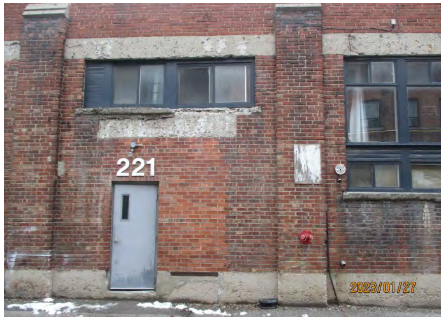
South elevation showing altered bay accommodating a smaller window and a door. Brick is heavily soiled below the cap stones above the pilasters and below window sills due to a lack of a proper drip edge below the cap stone.
