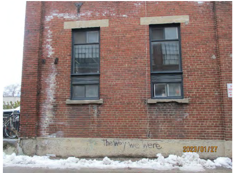
Building C (west) south elevation, showing weathered condition of brick wall, window sills and lintels, and concrete foundation. Of note is the heavy efflorescence near the corner. This efflorescence is also shown on the interior side, along with deteriorated masonry, likely due to faulty interior plumbing.
