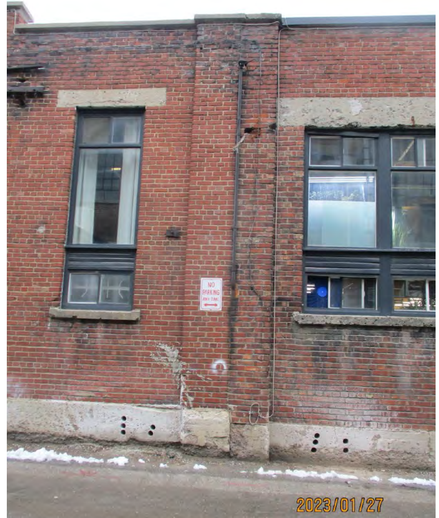
South elevation, at the junction between two construction periods (the western portion was built prior to the eastern portion) showing severely weathered brick parapet, localized corrosion staining at concrete lintel, weathered and heavily deteriorated window sills and brick staining due to water runoff and a lack of proper flashings or drip edges. Windows are wood and aluminum replacements (likely 1990s).
