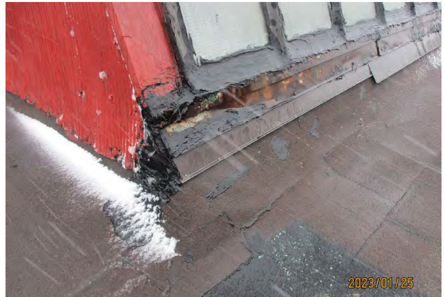
Close-up of a corner of a sawtooth skylight on the western portion of Building C. Note the heavy use of sealant throughout, which completely hides the steel frame profile. The bottom flashing is corroded and new flashing was added.
