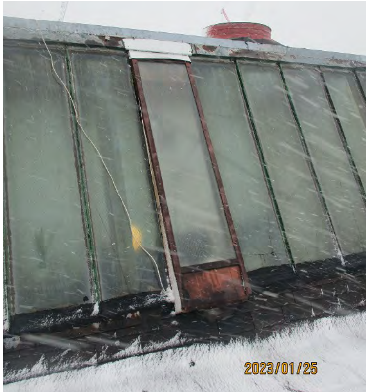
Close-up of a sawtooth skylight on the western portion of Building C. Note the fractured glass and sealants near the bottom of the frames. One window pane was altered with a new frame and appears to be crudely installed on the existing frame. The top flashing is rusted and appears to start deteriorating.
