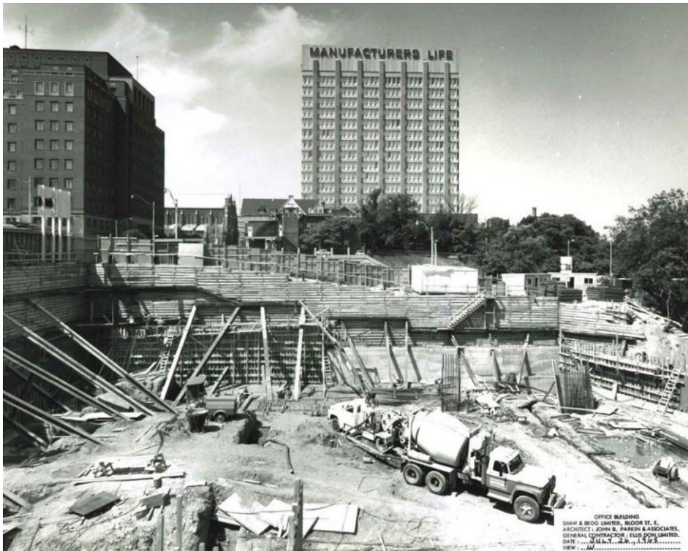
Image 23. 1968 photograph of Site during construction looking westward at the excavation area (Panda Associates).
