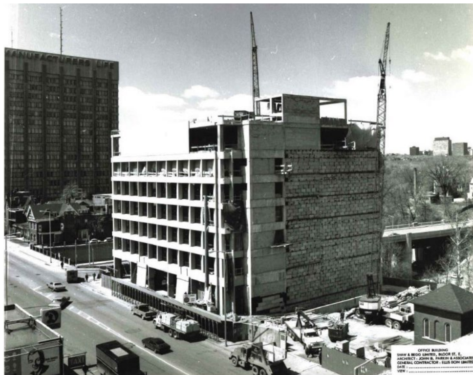
Image 26. c. 1969 photograph during construction, looking at the south and east elevations with the Mount Pleasant Bridge spanning Rosedale Valley Road and Ravine at right (Panda Associates).
