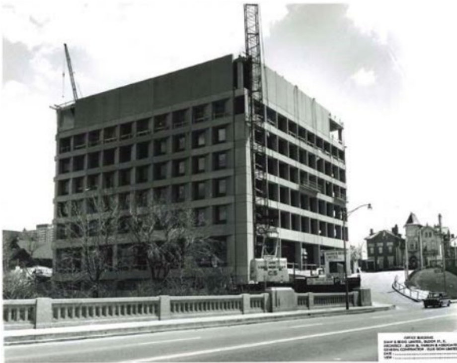
Image 29. 1969 photograph of Site during construction looking southeast and showing the property's interface with Bloor Street East elevated at background right and the ravine setting that falls away at left with the southern part of the Mount Pleasant Bridge in the foreground (Panda Associates).
