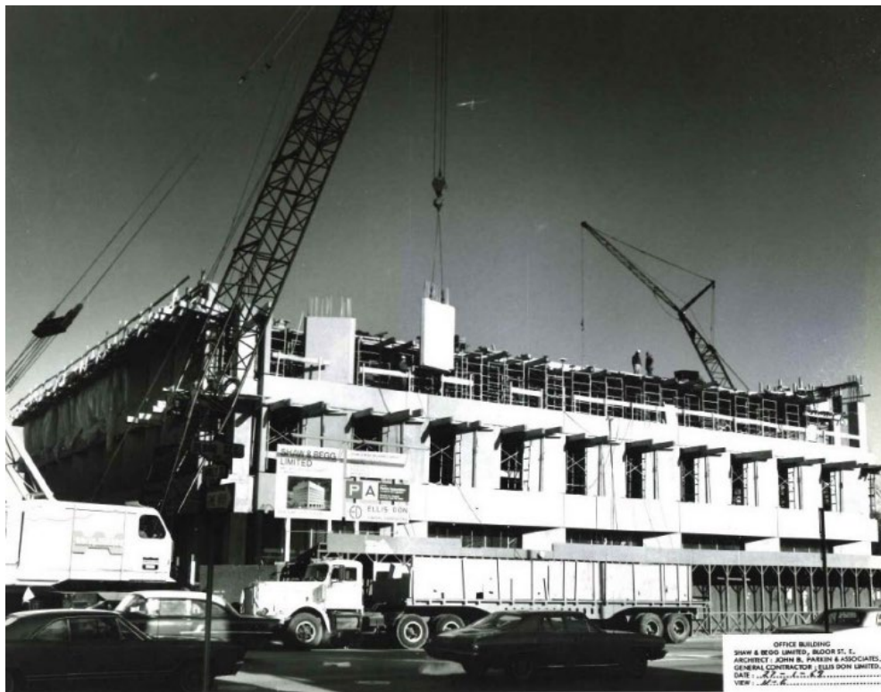
Image 25. 1969 photograph during construction, looking at the south and west elevations (Panda Associates).
