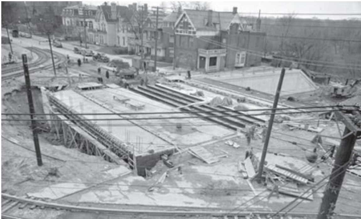
Image 10. 1946 aerial photograph looking northwest at construction of the Bloor Street underpass and Clifton Road Extension, later renamed Mount Pleasant Road, from south of Bloor Street East (Toronto Public Library).
