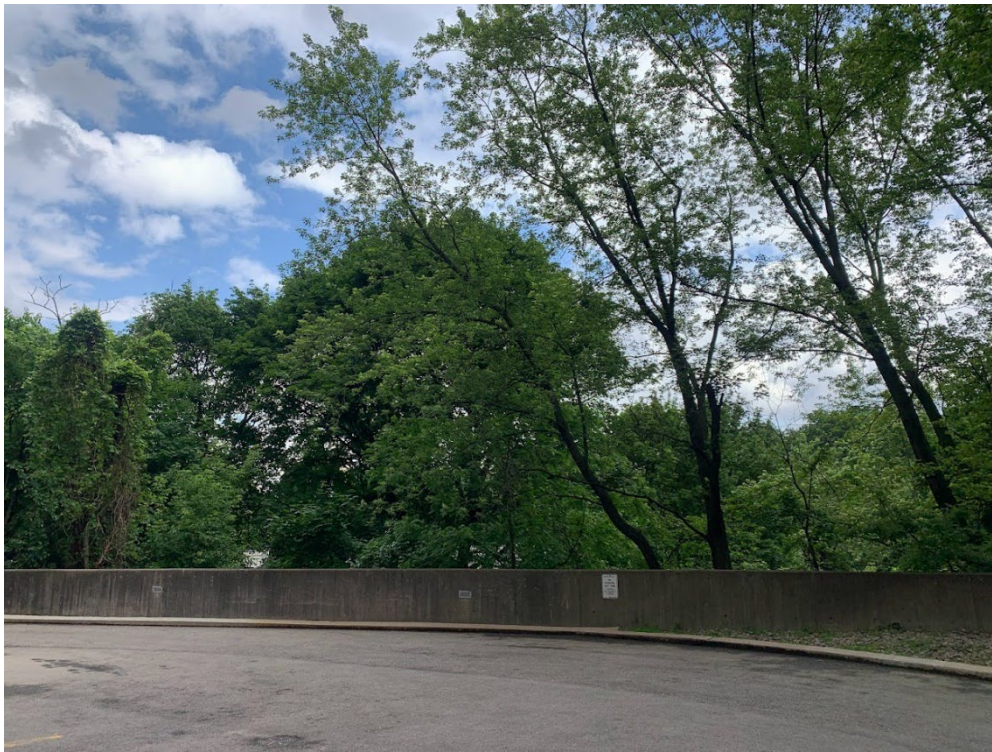
Image 44. Current photograph looking north at the interface between the concrete perimeter retaining wall of the site and the Rosedale Ravine beyond. (Heritage Planning, 2023)
