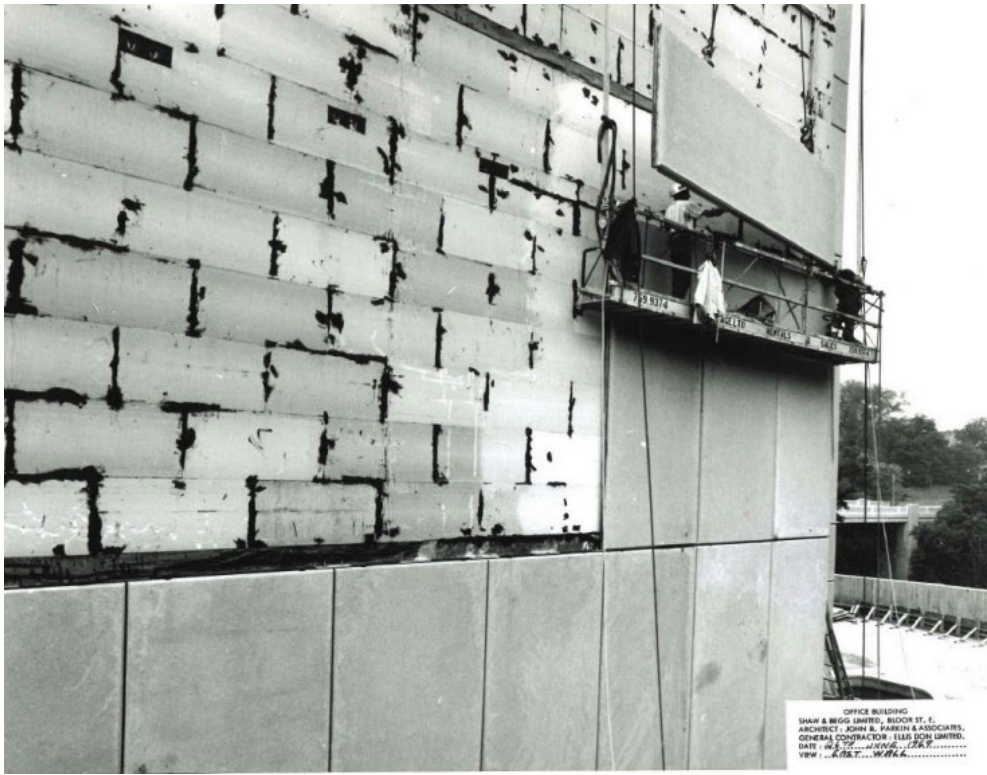
Image 27. 1969 photograph during construction, showing the installation of concrete panels on the largely blank east elevation (Panda Associates).
