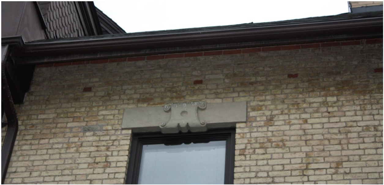
Figure 30. Detail of red brick and buff brick integration on 137 Bond Street, north elevation (Heritage Planning, 2023).
