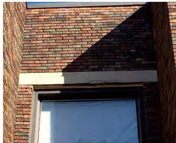
Fig.43: Efflorescence, recessed and missing mortar joints, west façade.
