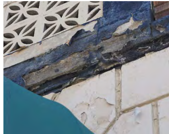
Fig.15: Example of peeling paint, spalling and deterioration on the lower cornice on the west façade.
