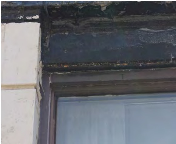
Fig.17: Example of holes and cracking in window sealant on the west façade.
