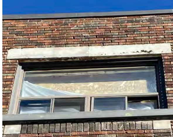
Fig.45: Peeling and cracked paint at cast stone lintels, west façade. Note recessed and open mortar joints above window, along with rust and peeling paint at lintel.
