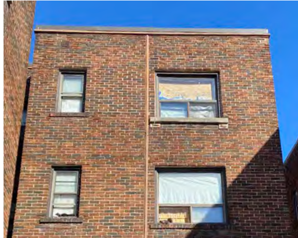
Fig.58: Typical condition of metal roof flashing, south façade.
