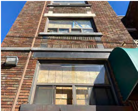
Fig.60: Typical condition of metal flashing over sills and banding, west façade.
