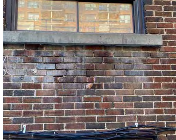
Fig.50: Poor condition of masonry below window, east façade. Note efflorescence, spalled masonry, stepped cracking and missing mortar joints.
