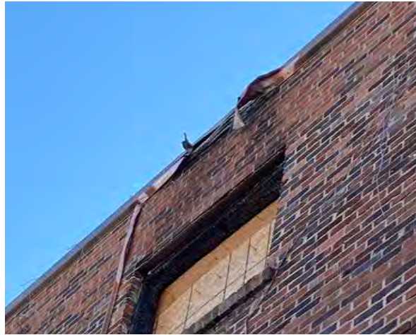
Fig.59: Defective area of metal roof flashing, east façade.
