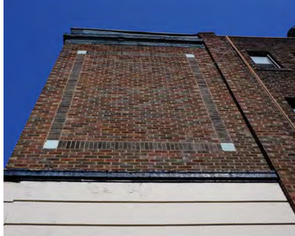
Fig.28: View of the upper and lower level cornices both with peeling paint on the south façade.
