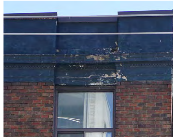
Fig.14: Example of peeling paint, spalling and deterioration on the upper cornice on the north side of the west façade.
