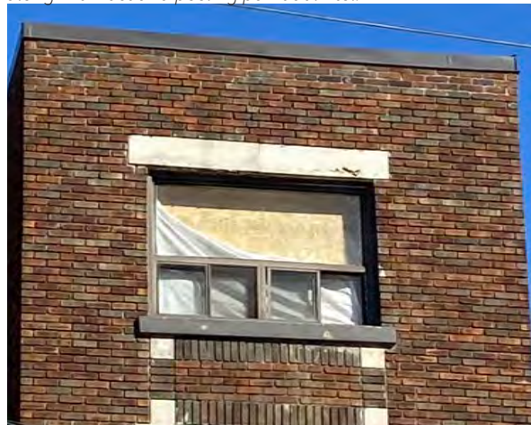
Fig.46: Typical masonry condition below roof line, west façade. Note selective masonry repointing, recessed and open mortar joints.
