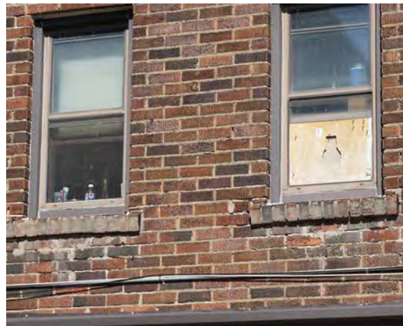
Fig.23: Example of poorly applied mortar repairs on the south façade.
