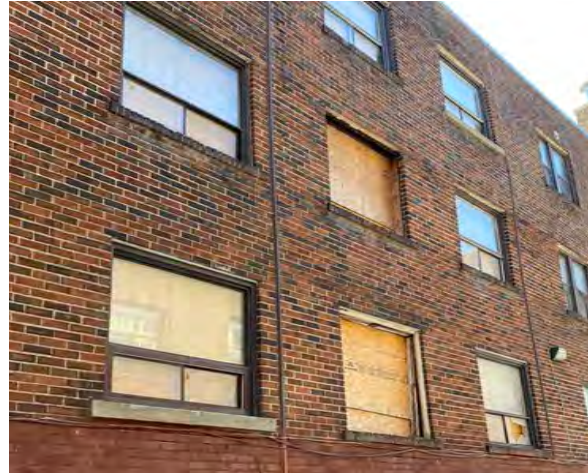
Fig.55: Typical condition of windows, north façade.
