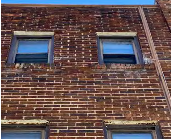
Fig.34: Example of sills with recessed and missing mortar joints on the north façade (March 2023).
