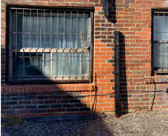
Fig.25: Mismatched masonry repairs at the base of the building on the south façade (March 2023).
