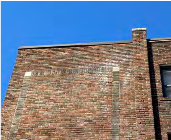
Fig.51: Condition of masonry, south façade. Note efflorescence, recessed and missing mortar joints.
