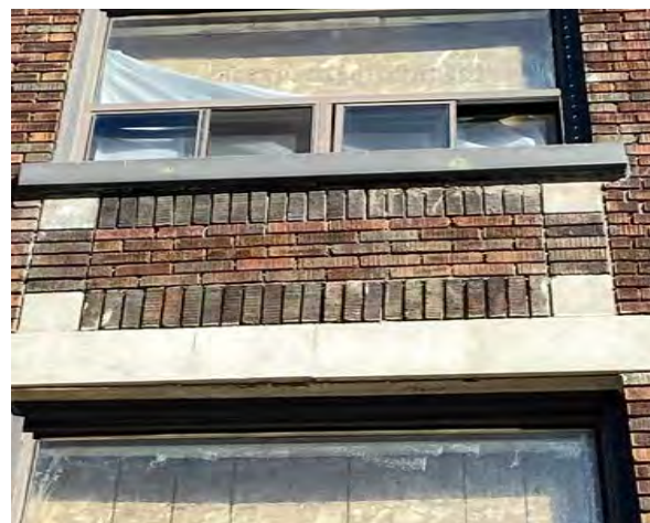
Fig.44: Typical masonry condition at decorative brick panels, west façade.
