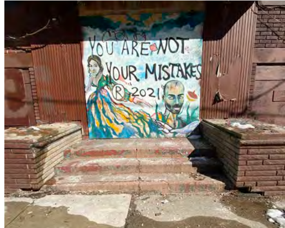
Fig.62: Condition of concrete steps at front entrance, west façade.
