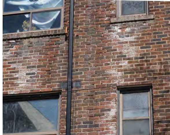
Fig.22: Example of efflorescence underneath windows on the south façade.
