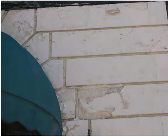
Fig.11: Example of the cast stone cladding where paint is peeling and the cast stone is spalling on the west façade.
