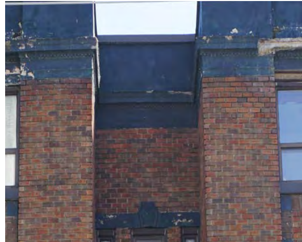
Fig.8: Example of light efflorescence, and recessed and missing mortar joints below the upper cornice on the west façade.
