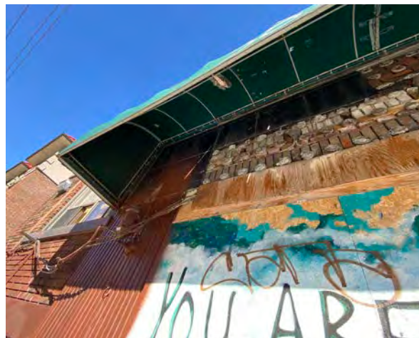
Fig.57: Exterior tiles in poor condition at entryway, west façade.
