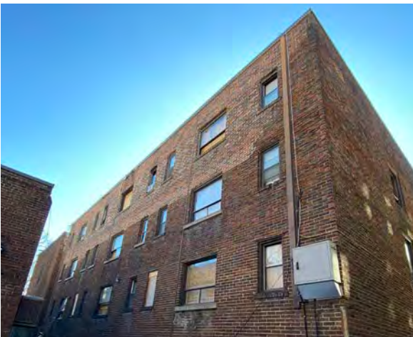
Fig.53: Mismatched repointing at top storey, east façade.
