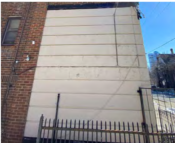
Fig.36: View of cast stone with peeling and cracked paint on the north façade (March 2023).
