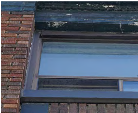
Fig.18: Example of window flashing with a dislodged panel on the west façade.
