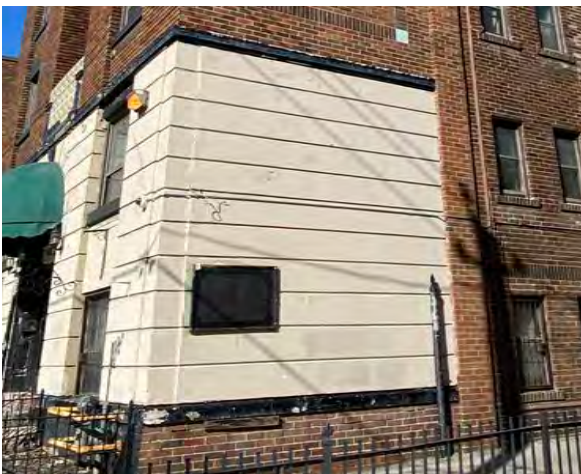
Fig.27: View of cast stone with peeling and cracked paint on the south façade (March 2023).
