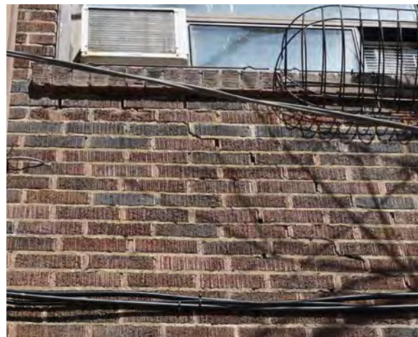
Fig.24: Example of step cracks under windows with air conditioning units on the south façade.
