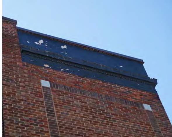
Fig.37: View of the peeling paint and spalling on cornice of the north façade.
