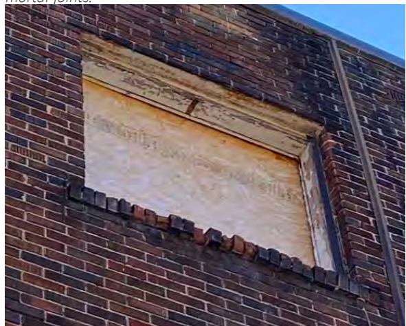
Fig.48: Poor condition of brick sills, north façade. Note rust and peeling paint at lintel.
