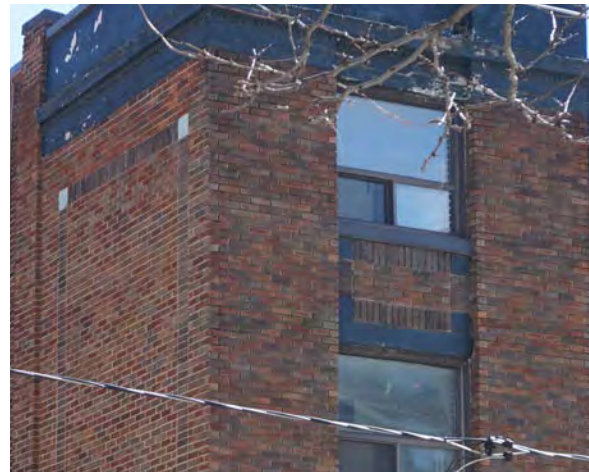
Fig.9: Example of recessed and missing mortar joints which run vertically along the corners on the west façade.
