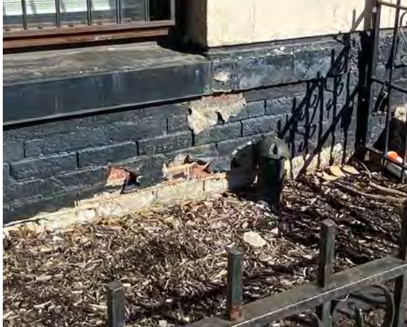
Fig.10: Example of painted brick at the base of the building with recessed mortar joints on the west façade.
