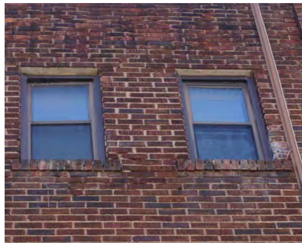
Fig.33: Efflorescence below window sills on the north façade.
