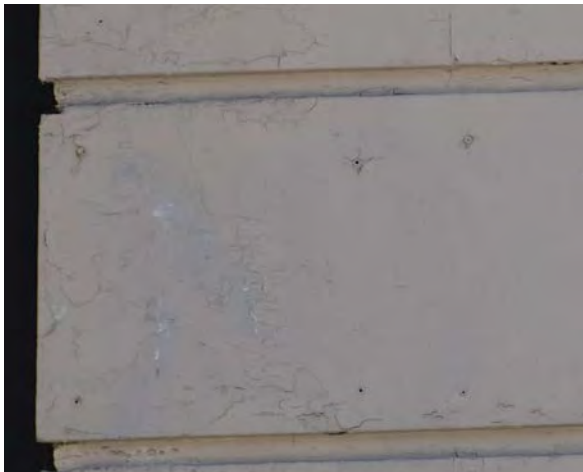
Fig.12: Example of holes in the cast stone panels on the west façade.
