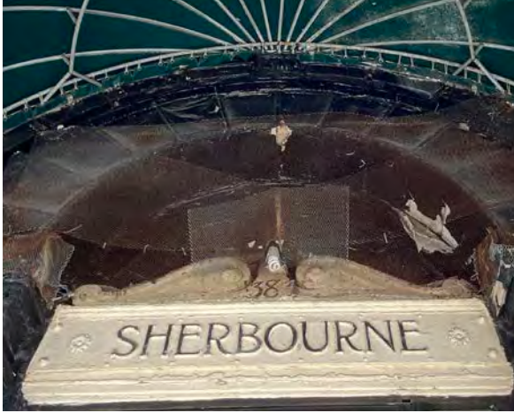
Fig.16: Condition of the ornamental lintel and the wood fanlight which has peeling paint and exposed wood on the west façade (March 2023).
