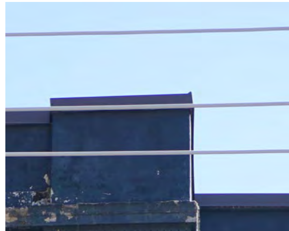
Fig.20: Example of roof flashing in good condition on the west façade.
