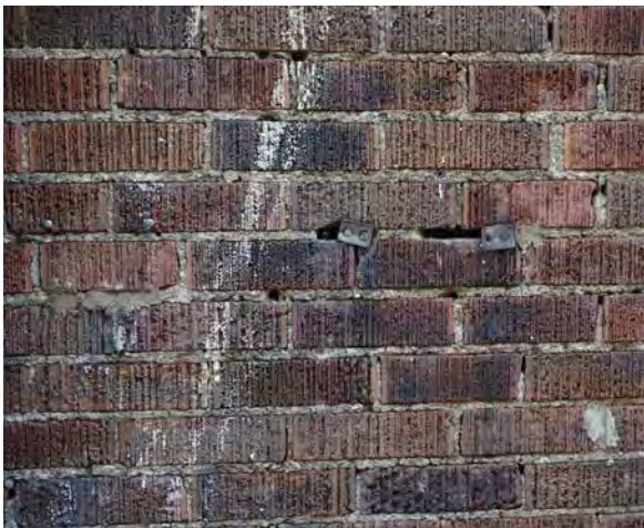
Fig.26: Example of holes in the masonry on the south façade.
