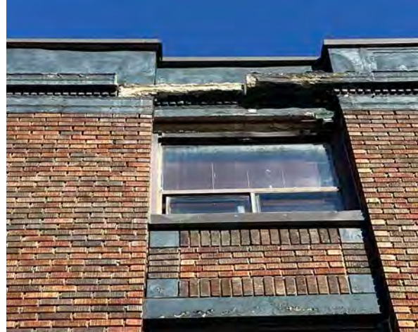
Fig.13: Example of peeling paint, spalling, deterioration on the upper cornice, south side of the west façade.
