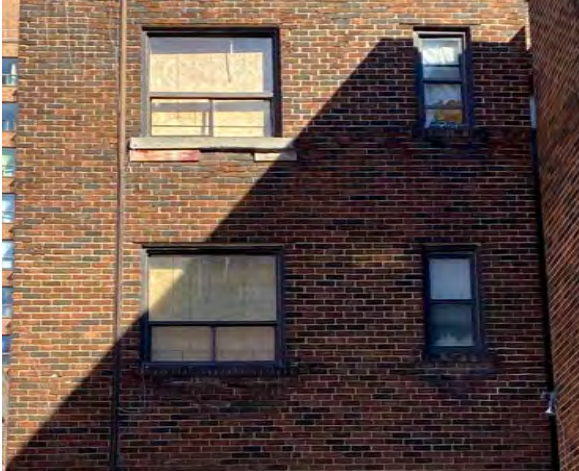
Fig.49: Poor condition of masonry below windows, north façade.
