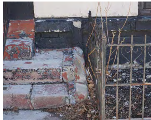
Fig.21: Example of concrete front steps with peeling paint and large cracks on the west façade.
