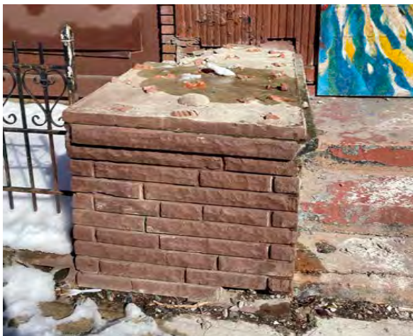
Fig.47: Condition at front entrance masonry pier, west façade.
