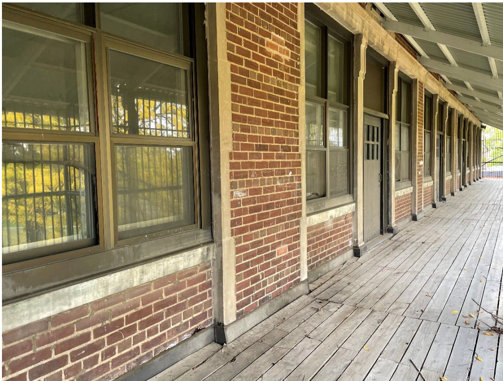
14. Balconies on the second storey of the south wing, extending the entire south elevation. Doorways permitted beds to be wheeled outside for heliotherapy (Heritage Planning, 2022)
