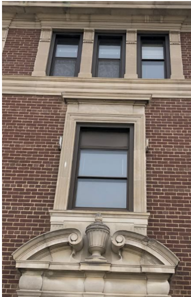
12. North façade details of the 2nd and 3rd storey windows (Heritage Planning, 2022)
