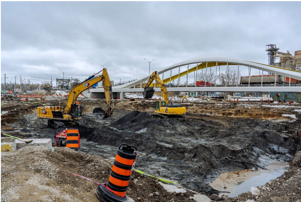
Excavation of the river valley, along the new Cherry Street (south) bridge as of winter 2023. Excavation is near the 'west plug' where the new river valley will connect to Polson Slip, becoming the new mouth of the Don River into Lake Ontario.
