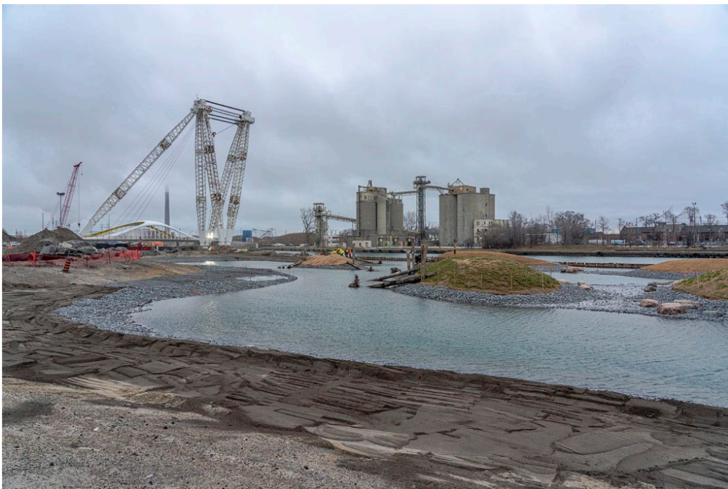
Construction of Canoe Cove, in Promontory Park South, looking southeast as of late fall/winter 2022. The restored Atlas Crane and the new Cherry Street (south) bridge is in the background.
