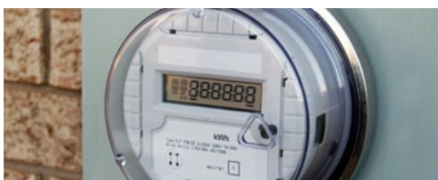
ADVANCED METERING FOR EV AND SOLAR INTEGRATION
