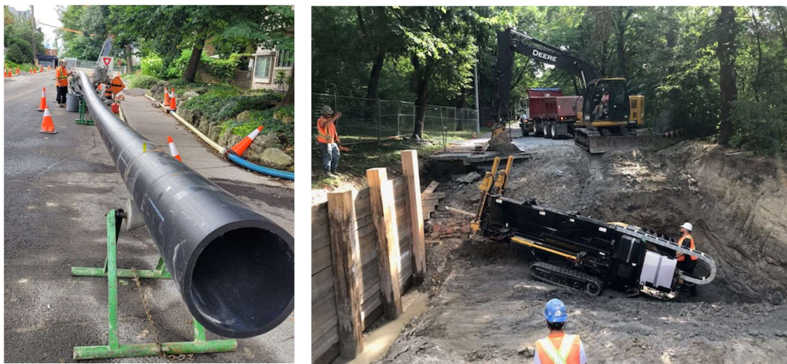
Figure 4 - HDPE Pipe Set-up on Ridge Dr and Directional Drill Set-Up on Carstowe Rd
