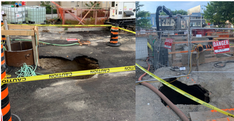
Figure 3: Sinkhole in the work zone between 1 and 2 Old Mill Drive
