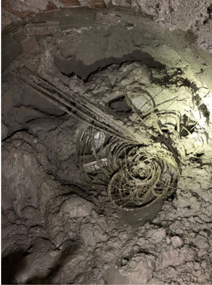
Figure 2: Face of the micro-tunnelling boring machine entangled in a steel tieback
