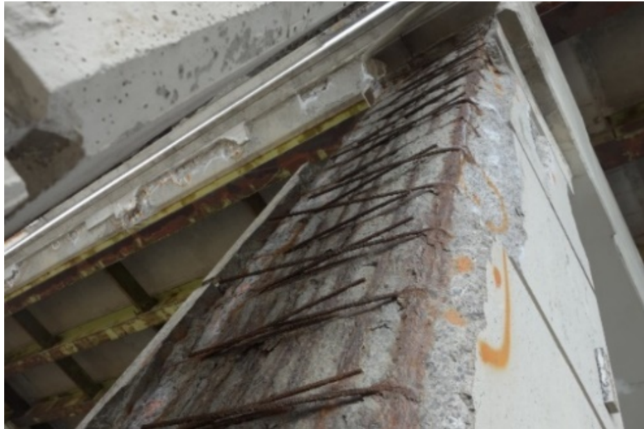
Figure 3: Condition of Reinforced Concrete Column at Bent 321
