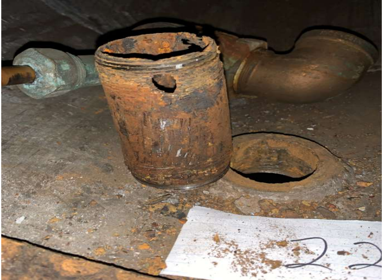
Figure 4 - Unforeseen Corrosion Conditions of a Drain Line Component
