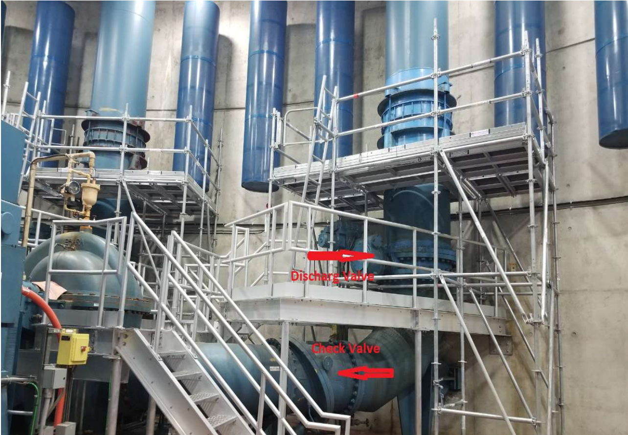
Figure 2 - Raw Water Pump Discharge Piping
