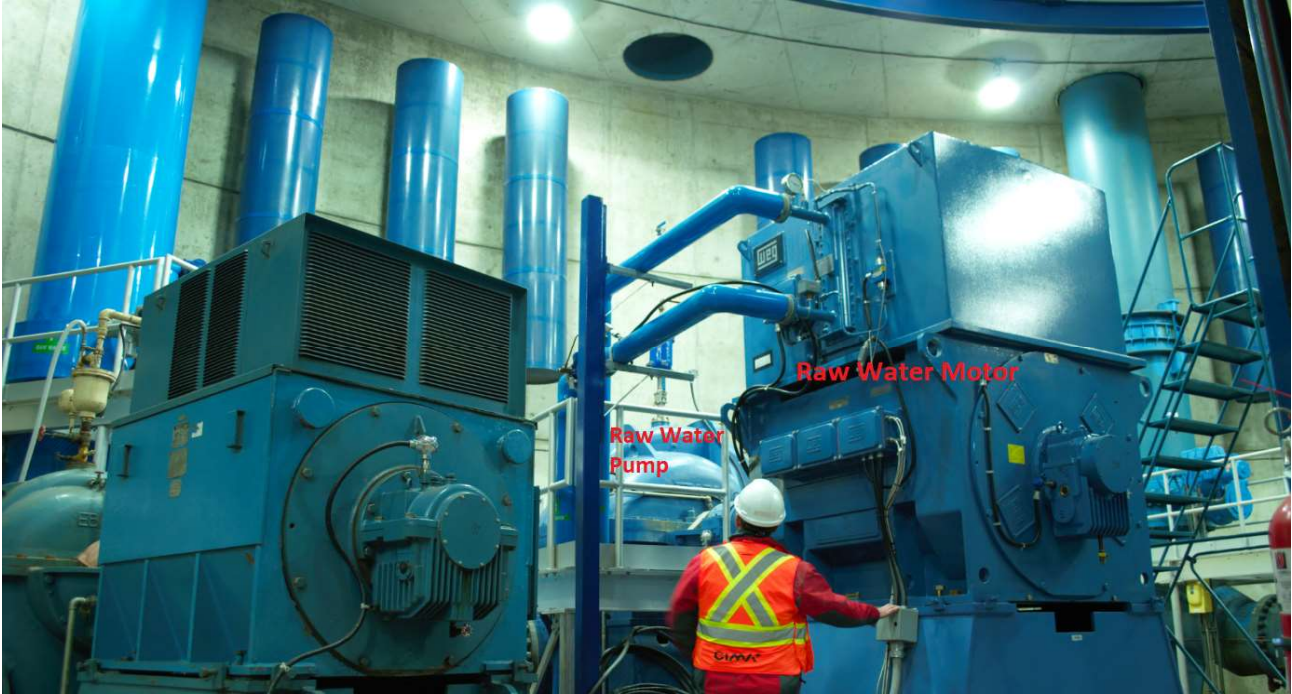
Figure 1 - Raw Water Pumps and Motors
