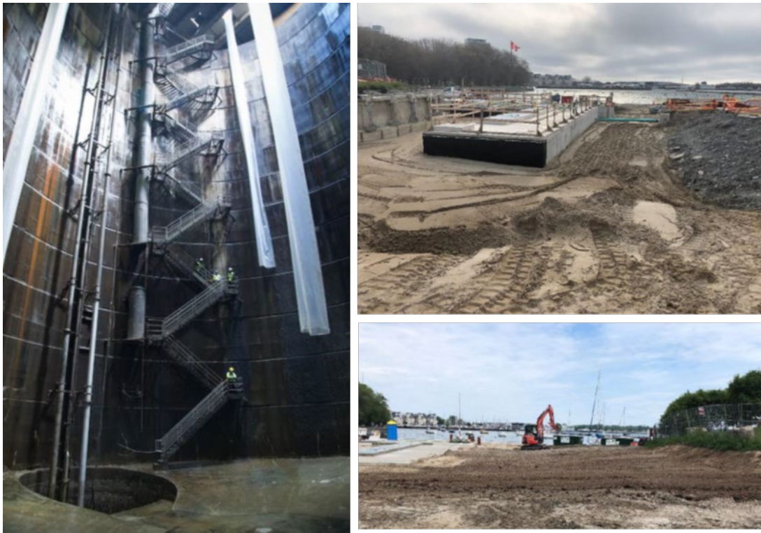
Figure 6: Left: Image of part of the Western Beaches Tunnel. Top right image of backfilling around the valve chamber for the Battery Park Interception Chamber. Bottom right image of final restoration work being completed for the Battery Park Interception Chamber
