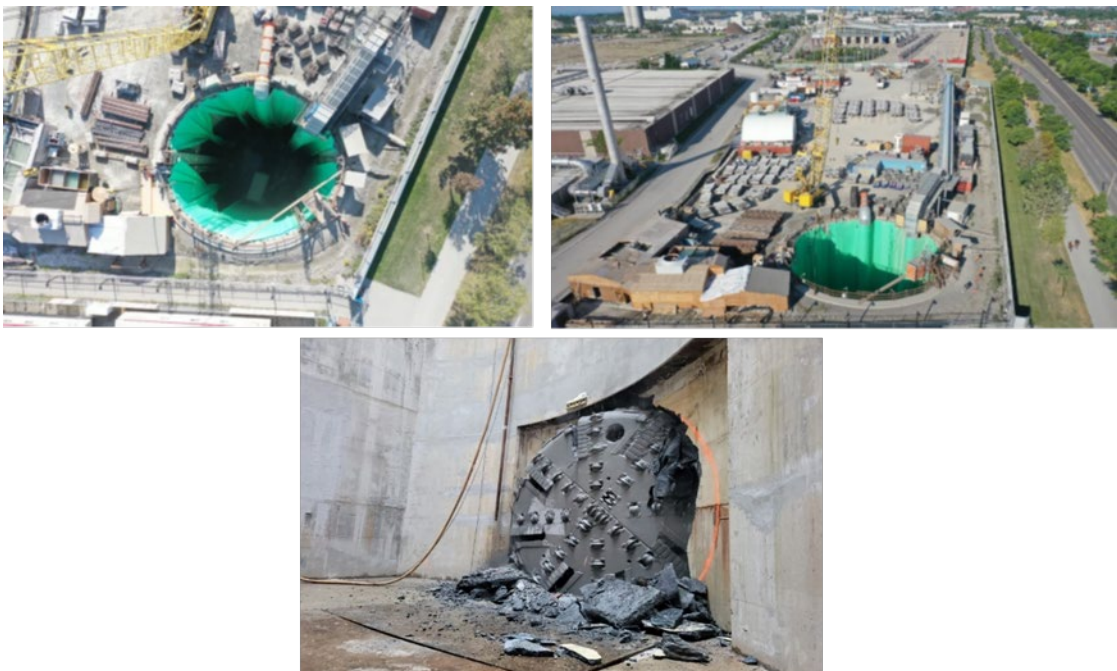
Figure 5: Top image of overhead views of the Coxwell By-pass tunnel. Bottom image of breakthrough of Tunnel Boring Machine for Stage 1 of Coxwell By-Pass in Summer 2022
