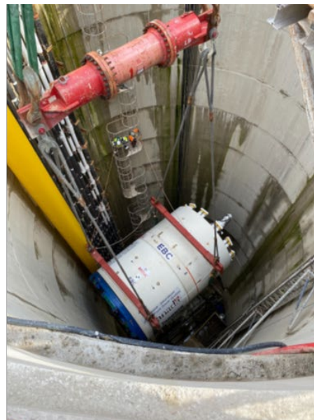
Figure 2: Left image of City officials and contractor in front of the 270-tonne Tunnel Boring Machine (named "Nabia") for the Fairbank Silverthorn Storm Trunk Sewer System project, which will work to construct a new storm sewer that will collect, store and move stormwater from the Fairbank-Silverthorn area to Black Creek to help reduce the risk of basement flooding. Right image Lowering of the tunnel boring machine into a
