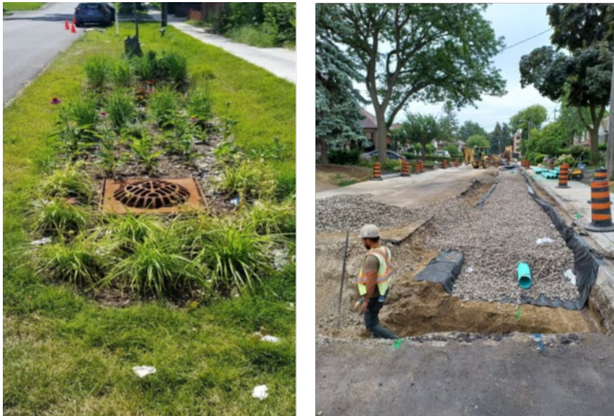
Figure 1: Left image of completed bioretention work as part of the Green Streets program on Byng Avenue. Right image of construction of green street work on Winnett Avenue (work was completed in August 2022)
