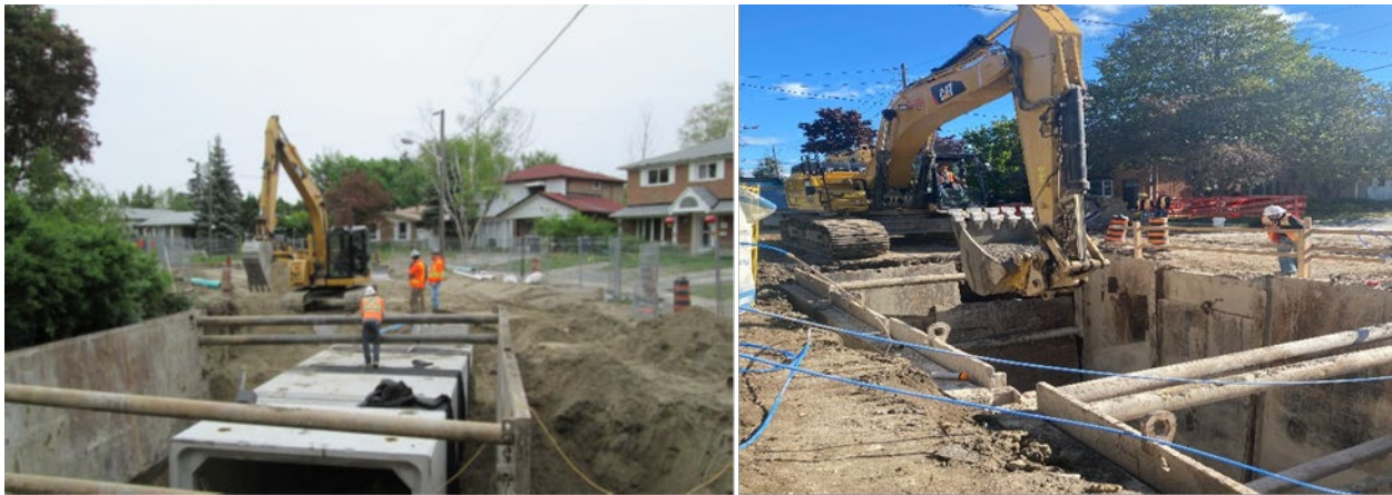
Figure 7: Left image of construction workers standing on new sewers being installed in a residential area as part of a basement flooding protection project. Right image of construction equipment backfilling a new sewer installation as part of the basement flooding protection program
