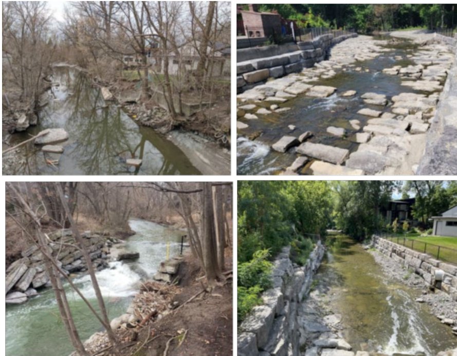
Figure 8: Images of Mimico Creek at Van Dusen Blvd Sanitary Sewer Protection – Top images look upstream before (left) and after (right) construction. Bottom images look downstream before (left) and after (right) construction.
