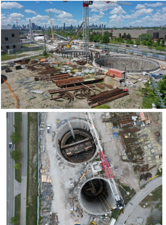
Figure 4: Top image of West-looking view of the integrated pumping station construction work site. Bottom image of overhead view of the wet weather flow and sanitary screen shafts at the integrated pumping station work site.
