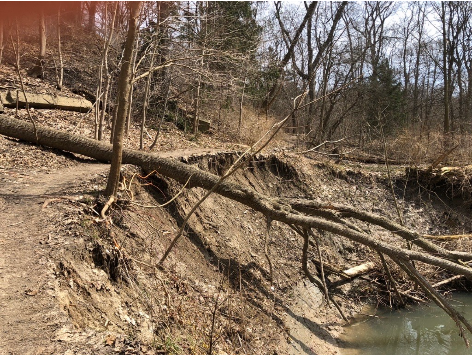
Erosion below Inglewood Avenue (Issue G on map)
