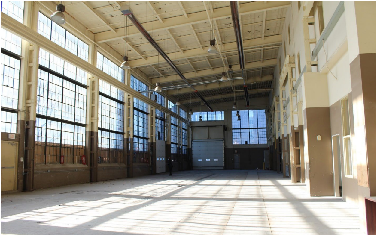
Figure 30: Interior photograph of 185 Eastern Avenue looking west, showing the south half of the building and large industrial window units along Palace Street. The interior demising wall that divides the building along the ridgeline of the roof is on the right of the photograph (SBA Ltd., 2021)
