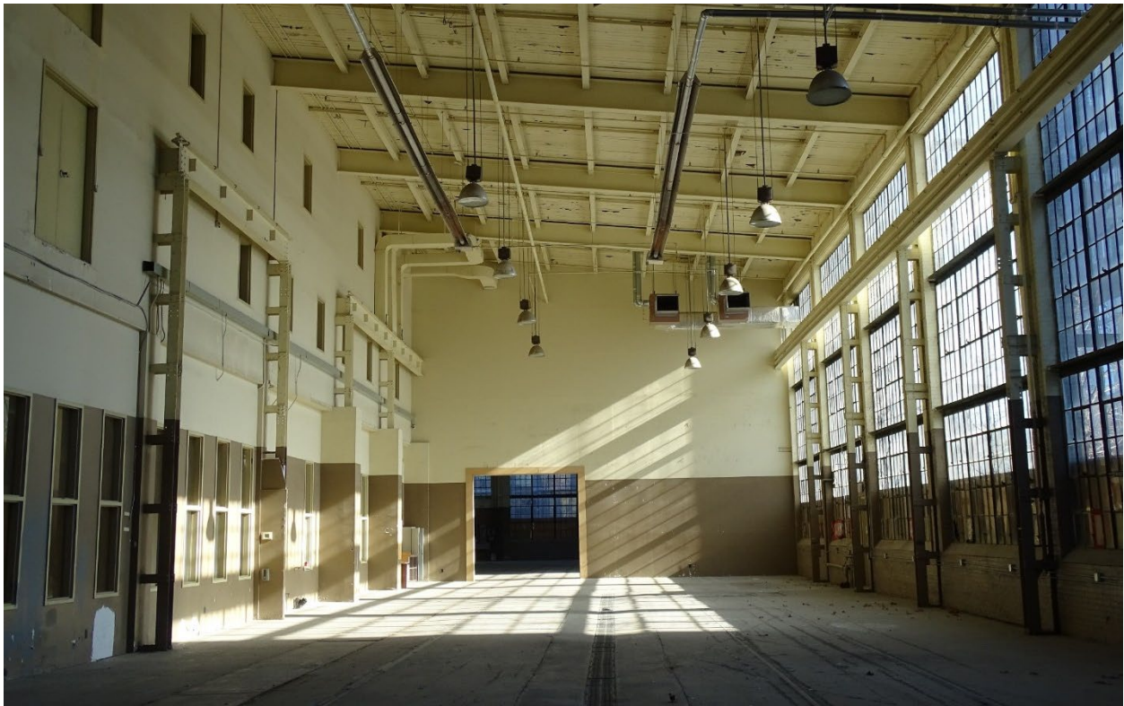
Figure 32: Interior photograph of 185 Eastern Avenue looking east, showing the south half of the building and large industrial window units along Palace Street. The interior demising wall that divides the building along the ridgeline of the roof is on the left of the photograph and the 1947 addition is visible through the large opening in the interior partition that divides the main space of the 1929 building. (SBA Ltd., 2021)
