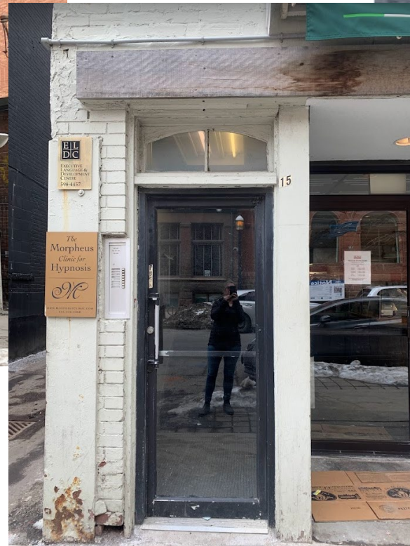
Early 1920s wooden door surround and transom on the principal (north) elevation
