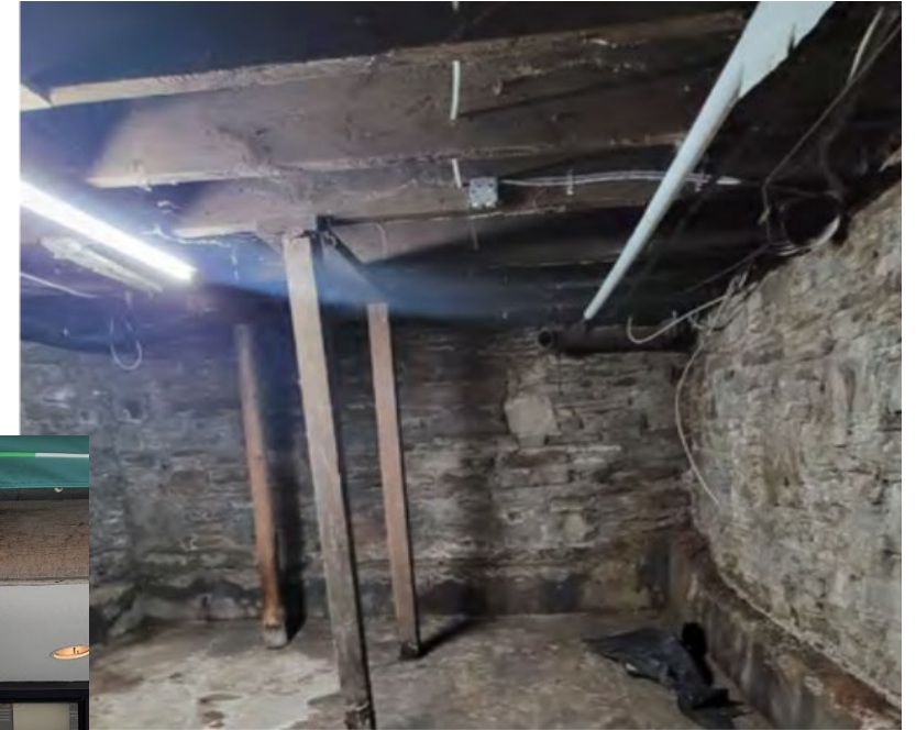
Basement interior at 15 Elm Street showing the rubble stone foundation and wooden cross beams
