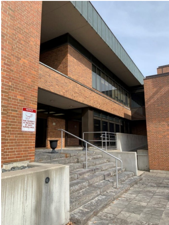
Figure 26. View of the primary entrance on the south elevation of the original 1962 office building showing the rough-hewn stone stairs, the concrete base, and the concrete ramp, looking northeast (Heritage Planning, 2023)
