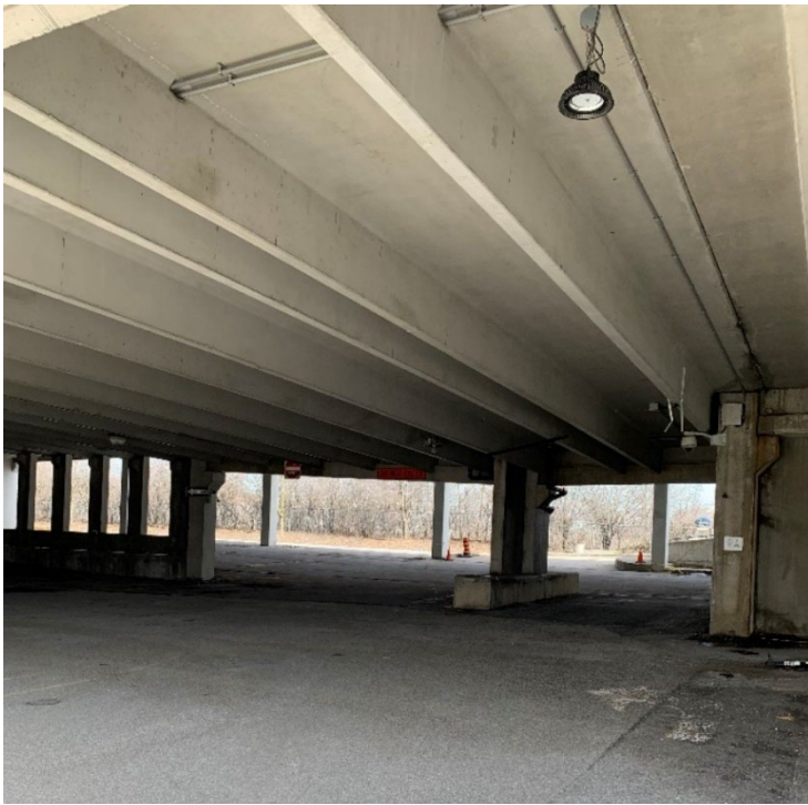
Figure 41. View of the two-storey parking garage constructed in 2006-2007, looking east (Heritage Planning, 2023)
