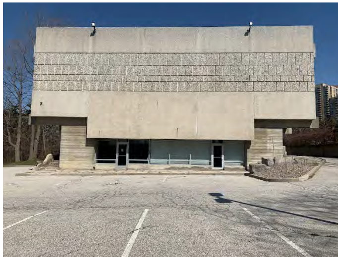
44. Current photo showing the south elevation with its four courses of coarse aggregate pre-cast concrete panel banding, 2023 (Heritage Planning)
