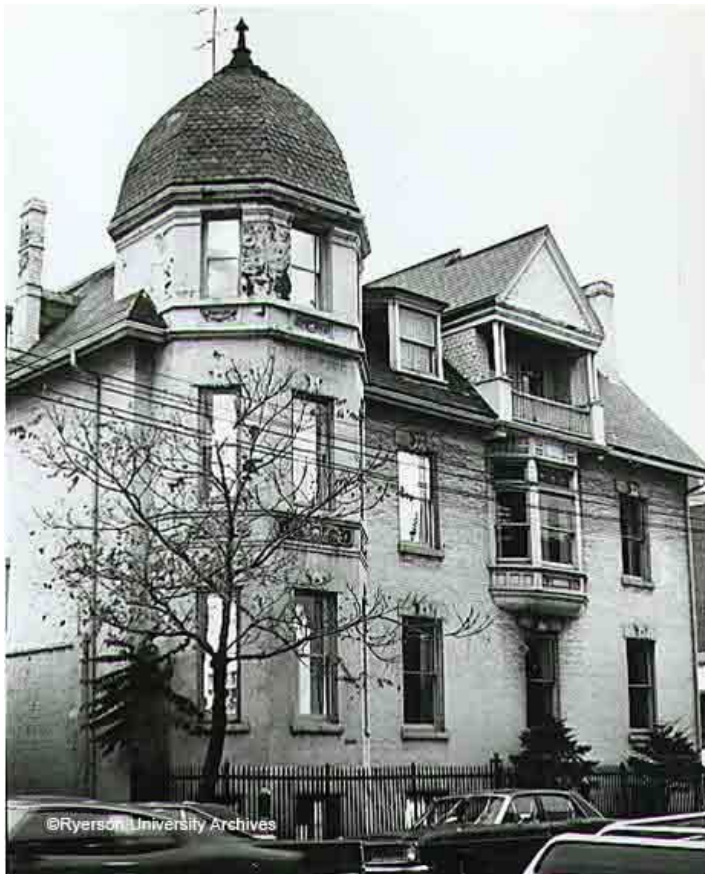
Figure 17. View of 137 Bond Street's north elevation showing peeling paint on third storey of turret, 1974 (photograph by Olga Cyhanenko, TMU Archives, retrieved from https://library.torontomu.ca/asc/2018/09/ryerson-7025-student-housing/ )
