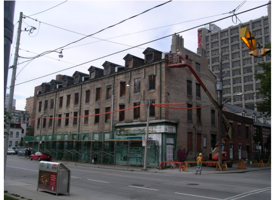
Photo HPS, 2006. The building collapsed in 2007 after years of neglect.
