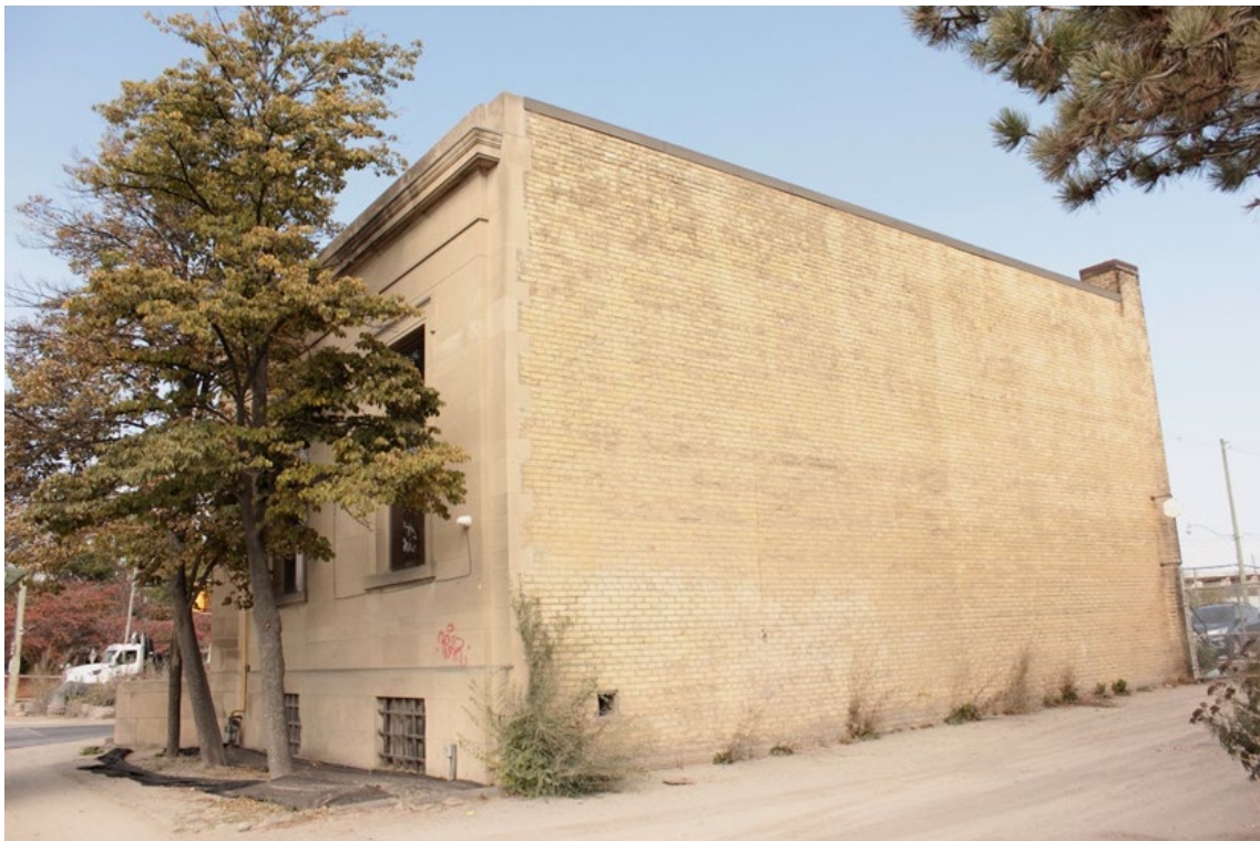
Figure 18. At top: east elevation and at bottom: south elevation of the former Bank of Montreal (Heritage Planning, 2023).
