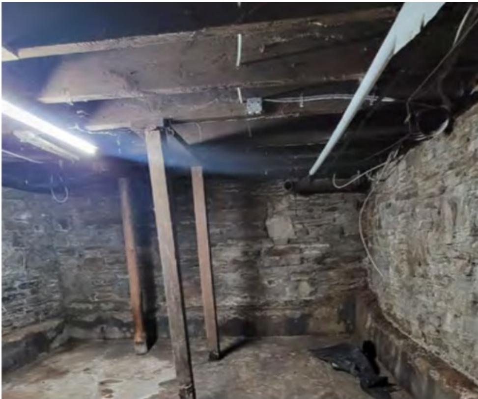
Image 19. Current photo of the basement interior at 15 Elm Street showing the rubble stone foundation and wooden cross beams (ERA, 2022)
