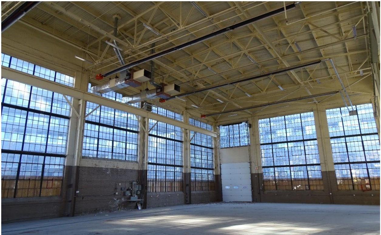
Figure 33: Interior photograph of 185 Eastern Avenue showing the eastern addition including steel roof trusses and gantry crane support structure, looking southeast (SBA Ltd., 2021)
