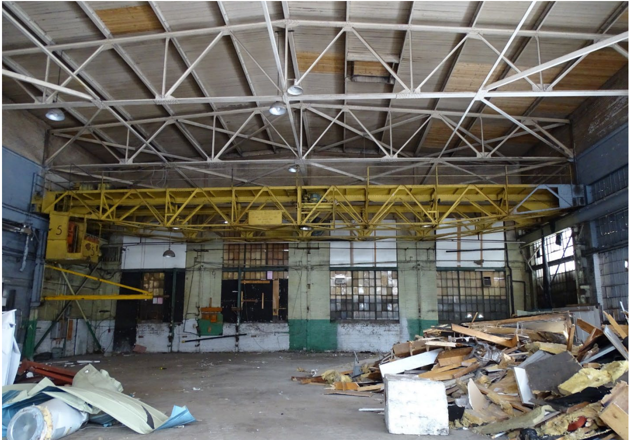
Figure 40: Interior photograph of 153 Eastern Avenue, showing the steel roof trusses, wood roof decking, and the steel gantry crane with secondary support structure. (SBA Ltd., 2021)
