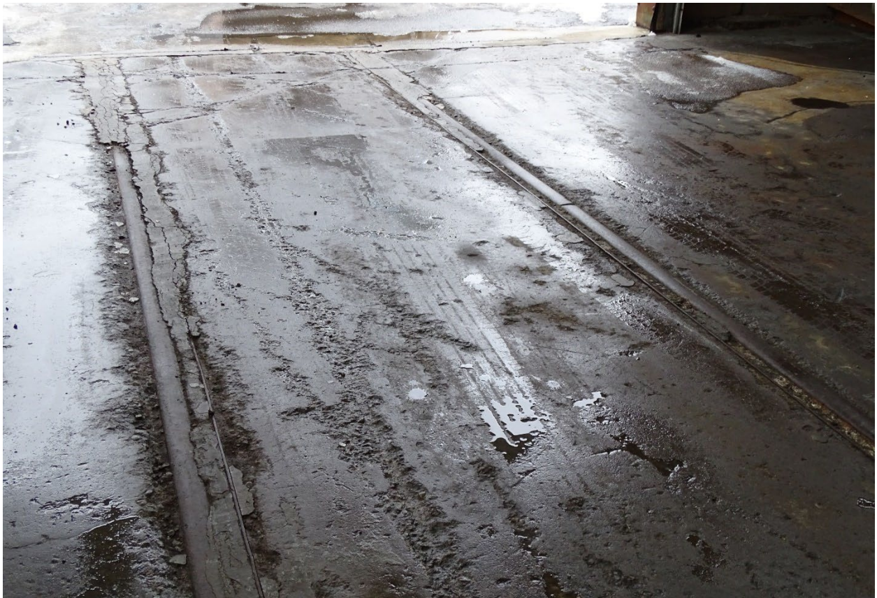
Figure 34: Interior photograph of 185 Eastern Avenue showing the detail of the railway tracks embedded in the concrete floor slab (SBA Ltd., 2021)
