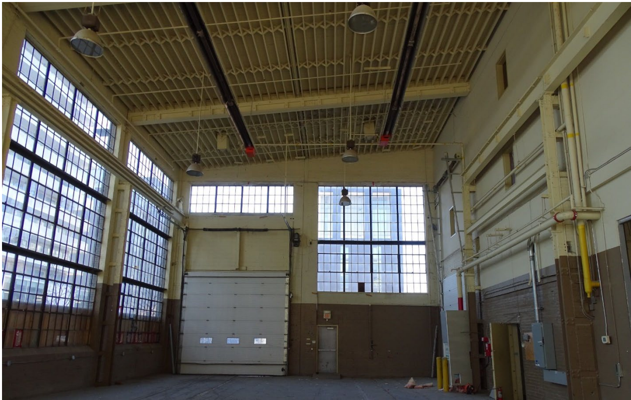
Figure 31: Interior photograph of 185 Eastern Avenue looking west, showing a closer detail of the roof structure in the western addition (SBA Ltd., 2021)
