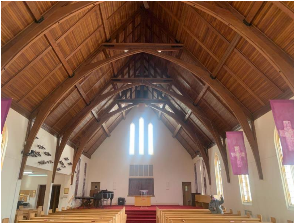
Image 39. Looking east across the nave to the sanctuary with raised platform and the 1962 additional (easternmost) bay seamlessly integrated with the 1947 design. (Heritage planning, 2023)
