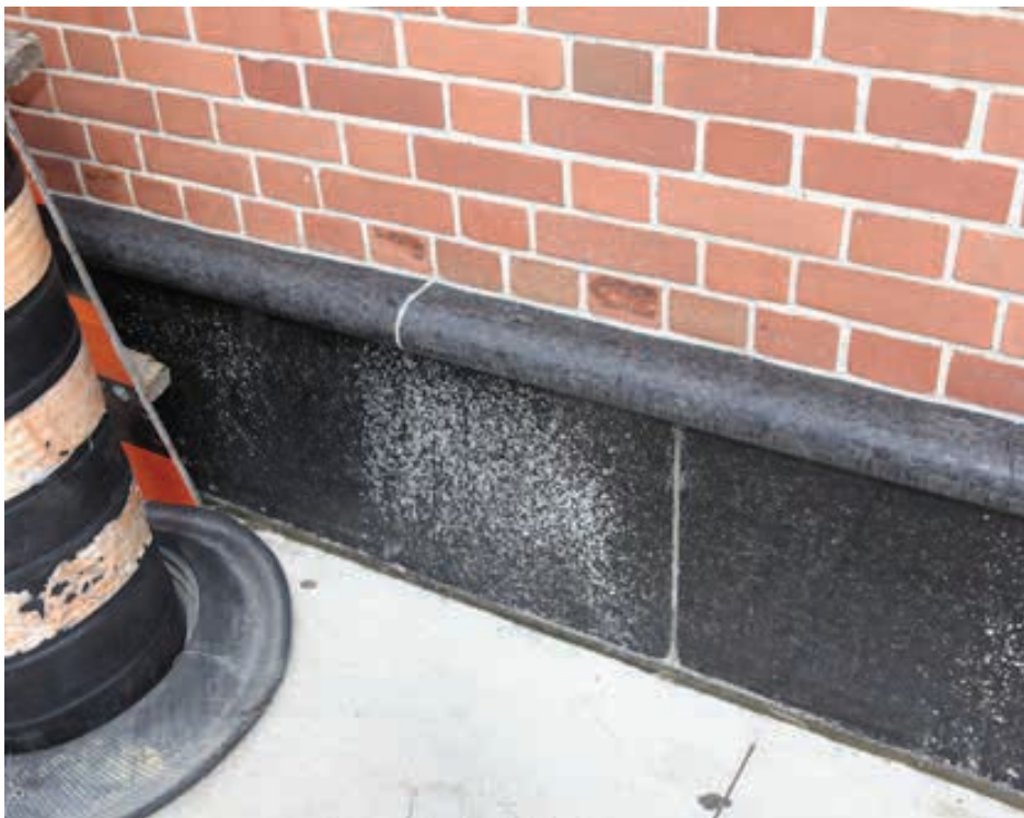
Image 49. Detail of the black granite plinth at the base of the north and west elevations (ERA, 2021)
