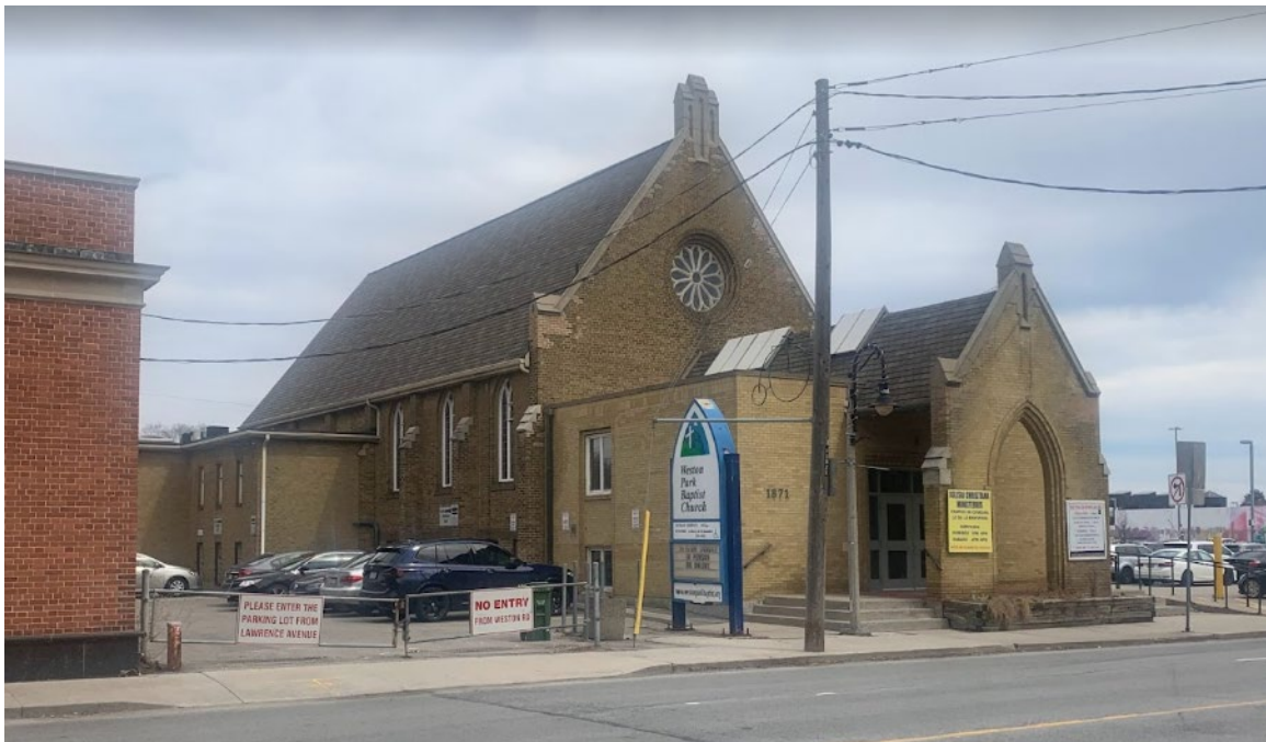
Image 31. Looking southeast at the north elevation of the nave and 1983-1984 rectangular vestibule fronted by the reconstructed 1947 vestibule façade. Part of the 1962 rear wing is also visible at left (Heritage Planning, 2023)
