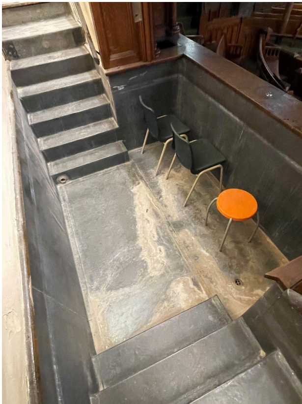
Figure 25: Detail view showing the lined baptismal tank at the West wall of the Sanctuary, 2022 (City of Toronto Heritage Planning)
