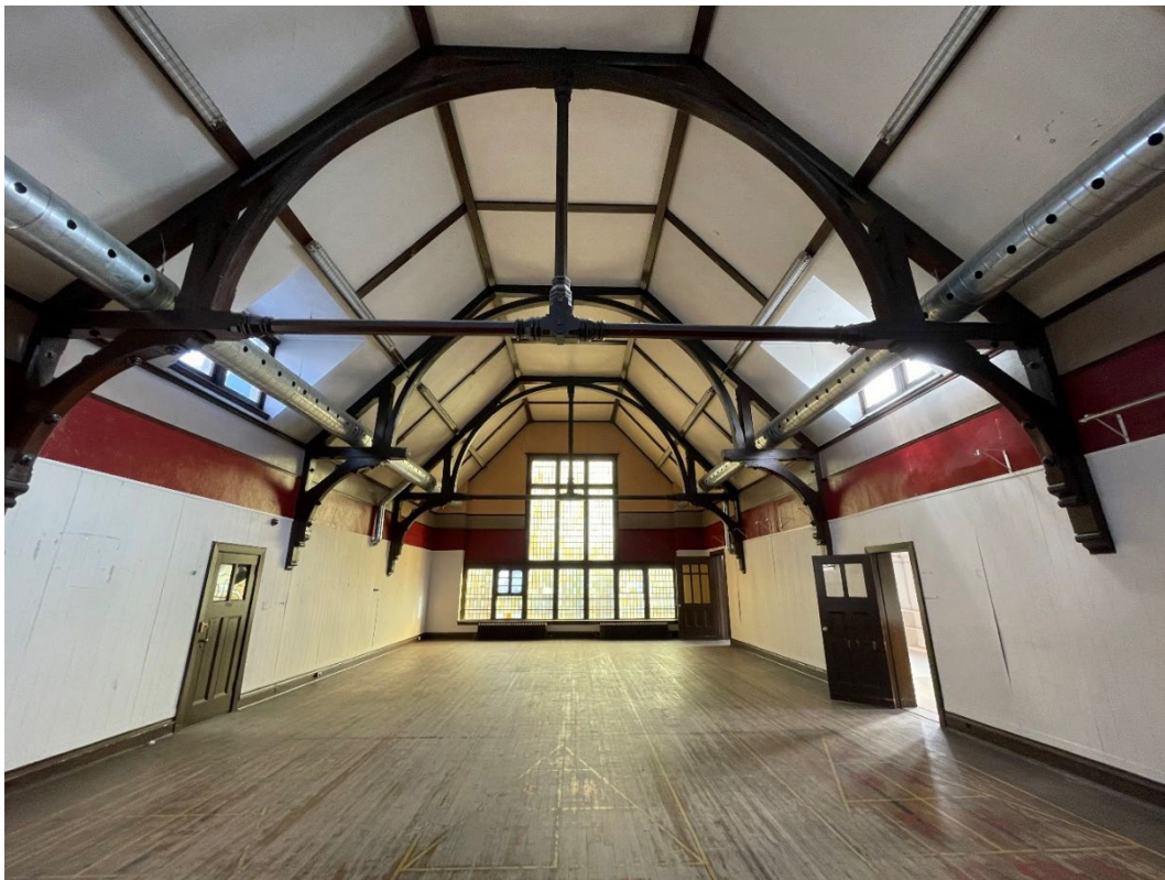
Figure 11: Interior upper level of the Sunday School Building showing the open truss, ceiling, 2022 (City of Toronto Heritage Planning)
