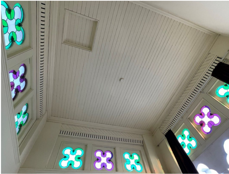
Figure 12: Interior of the Sunday School Building showing the interior of the tower, 2022 (City of Toronto Heritage Planning)
