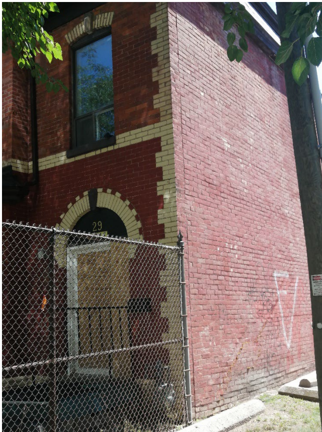
Figure 22 Northwest corner of 29 Linden Street. Note running masonry joint from later addition of brick cladding to the west elevation (Heritage Planning, 2023).
