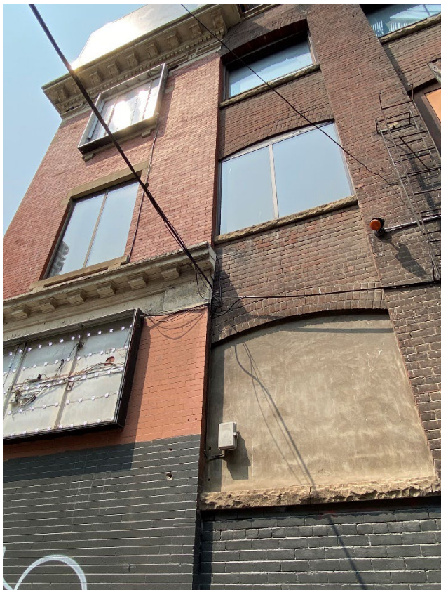
15. South elevation showing the architectural details of west (principal) elevation including the cornice continue/return to the first bay (Heritage Planning, 2023)
