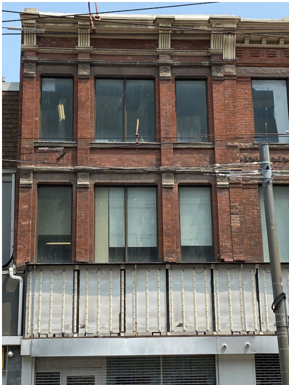
17. West (principal) elevation of entrance address 123 Church Street showing a late-Victorian architectural style (Heritage Planning, 2023)
