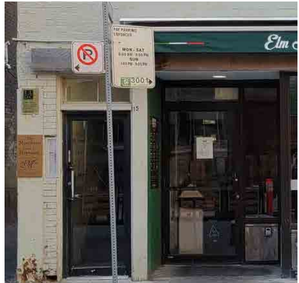
Figure 45: Second floor aluminium door with heavy steel angle and deteriorated brick in poor condition (ERA, 2022).
