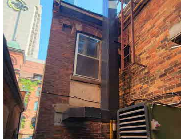
Figure 50: Open masonry with wood infill and windows ranging from poor to defective (ERA, 2022).
