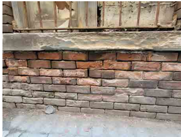
Figure 68: Spalled brick and damaged sills have no mortar, allowing water to enter the wall (ERA, 2022).
