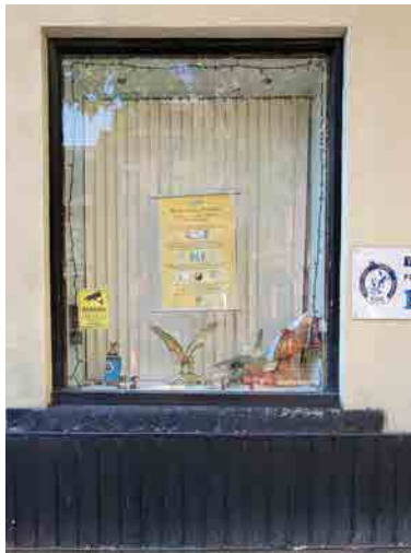
Figure 64: Black metal flashing and a painted stone sill in poor condition (ERA, 2022).
