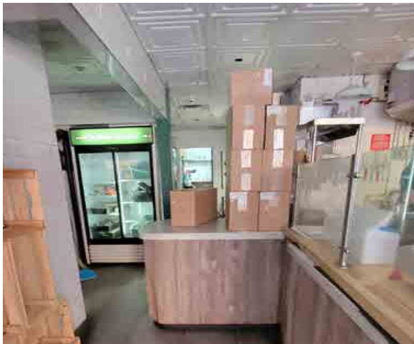
Figure 60: Restaurant interior in fair condition (ERA, 2022).
