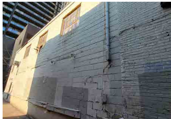
Figure 49: Rear steel windows are defective with rust and cracked panes (ERA, 2022).
