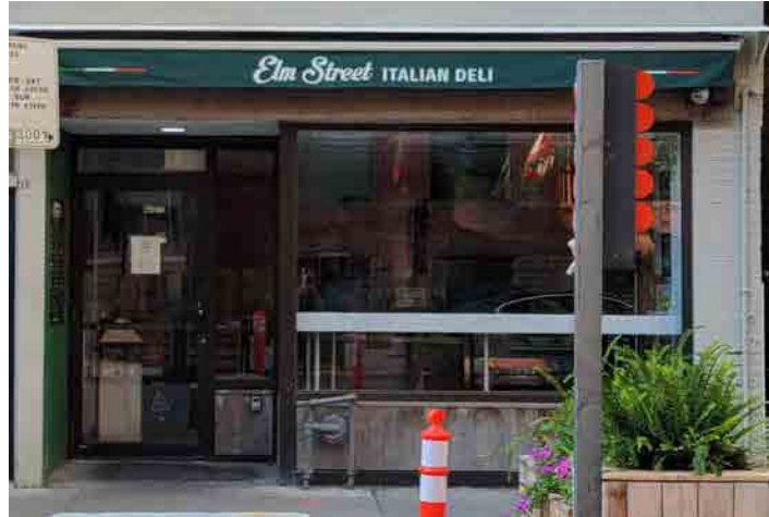
Figure 43: Aluminium storefront with glazing in poor condition (ERA, 2022).
