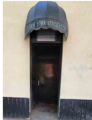
Figure 66: Separate entrance with steel door in poor condition (ERA, 2022).
