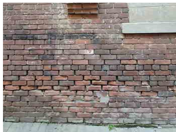
Figure 70: Mortar loss and defective masonry on the east elevation (ERA, 2022).
