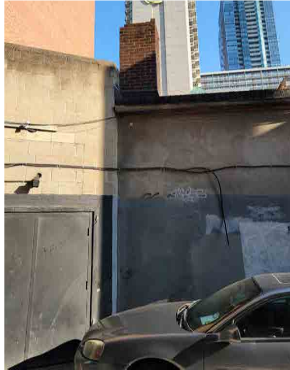
Figure 71: The south east corner is in poor condition (ERA, 2022).
