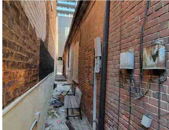
Figure 67: Areas of the east brick wall and concrete block infill is in defective condition (ERA, 2022).
