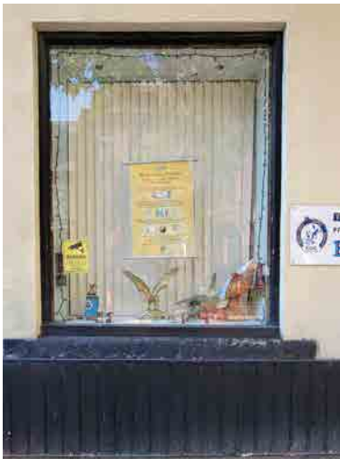
Figure 64: Black metal flashing and a painted stone sill in poor condition (ERA, 2022).
