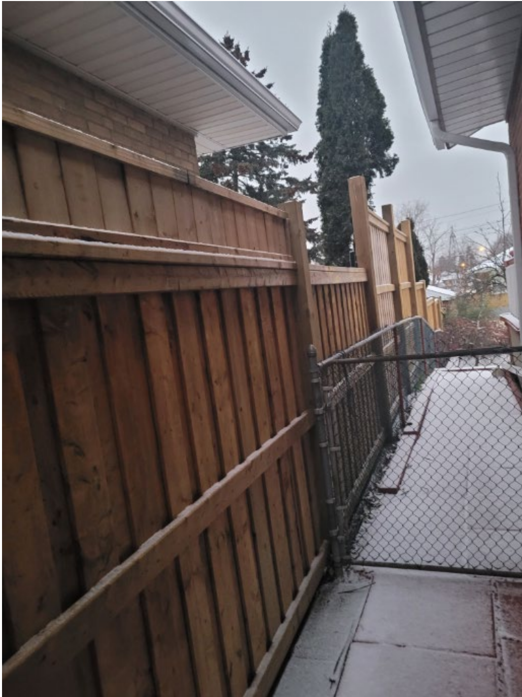
Attachment 3: Photo of fence from neighboring property
