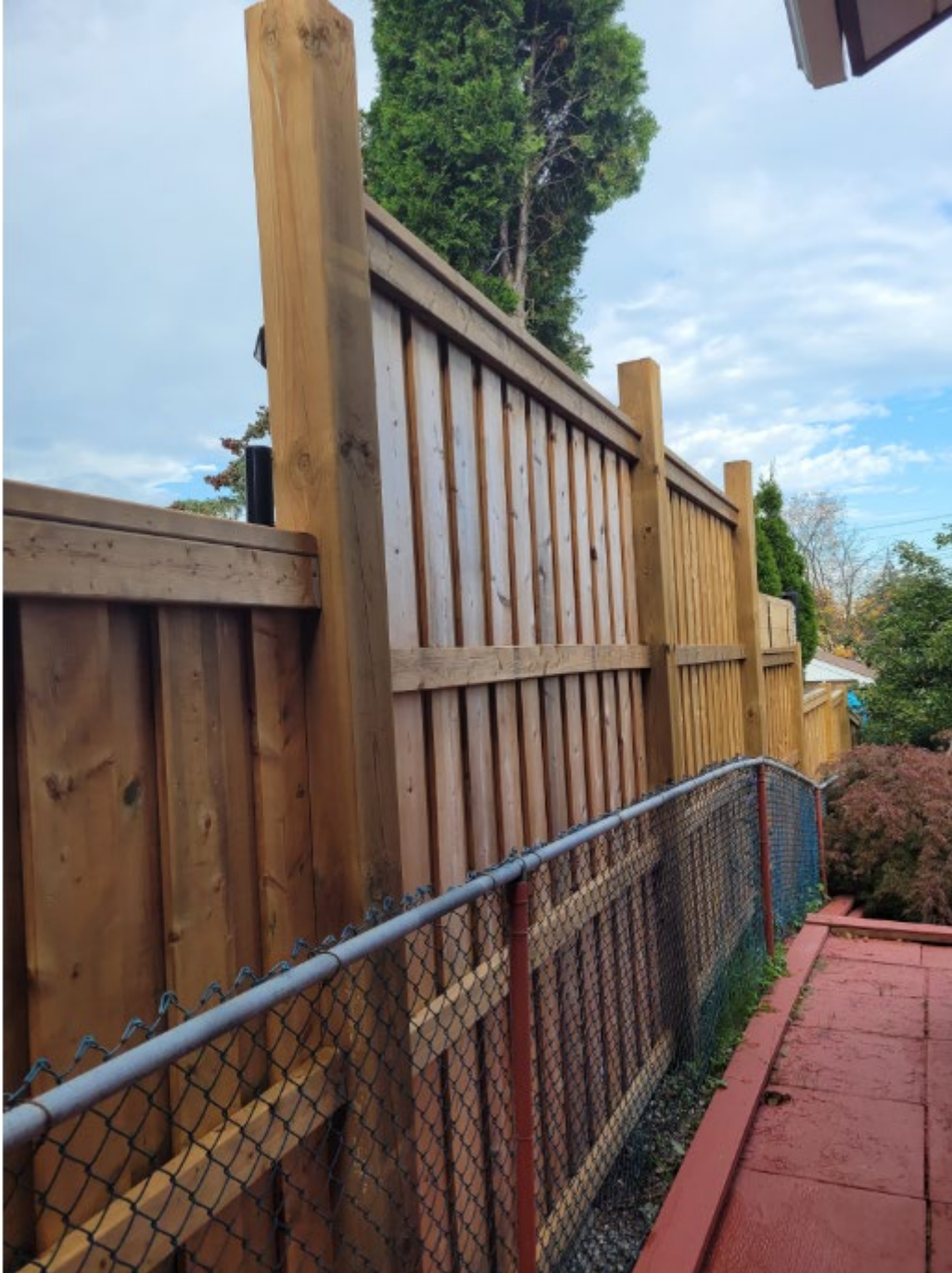
Attachment 2: Photo of fence from neighboring property
