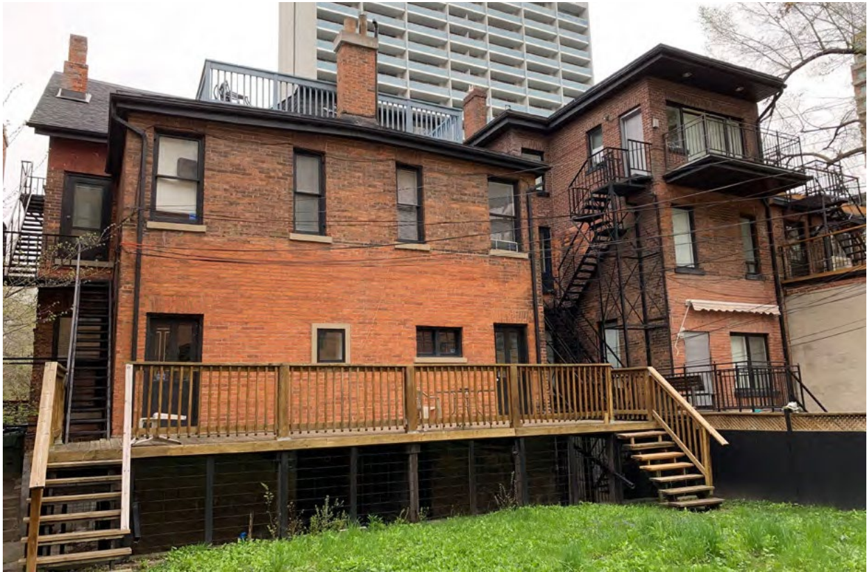
Rear (south) elevation of 29-31 Prince Arthur Avenue showing existing rear additions to be removed. (ERA Architects, 2022)
