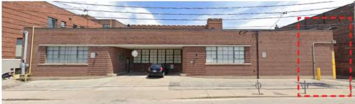
Front façade of 41 Fraser Avenue with approximate 3m area of wall to be removed highlighted in red (ERA Architects)
