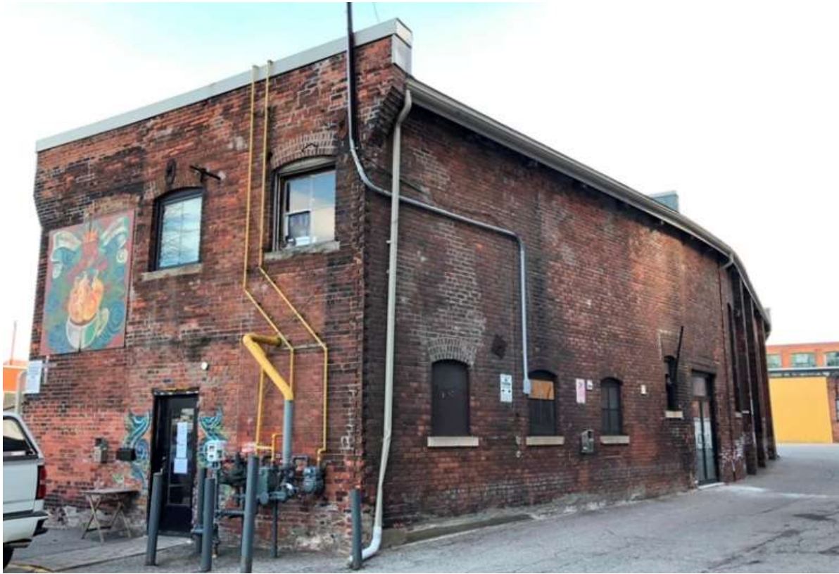
North and west facades of the powerhouse building showing the angled wall which was altered to accommodate the railway spur (HP, 2020)
