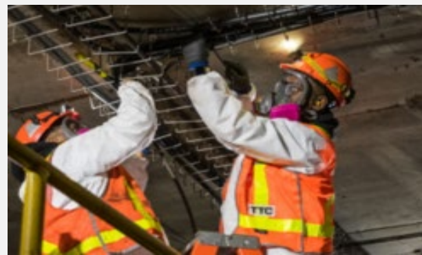
Network Wide Asset
