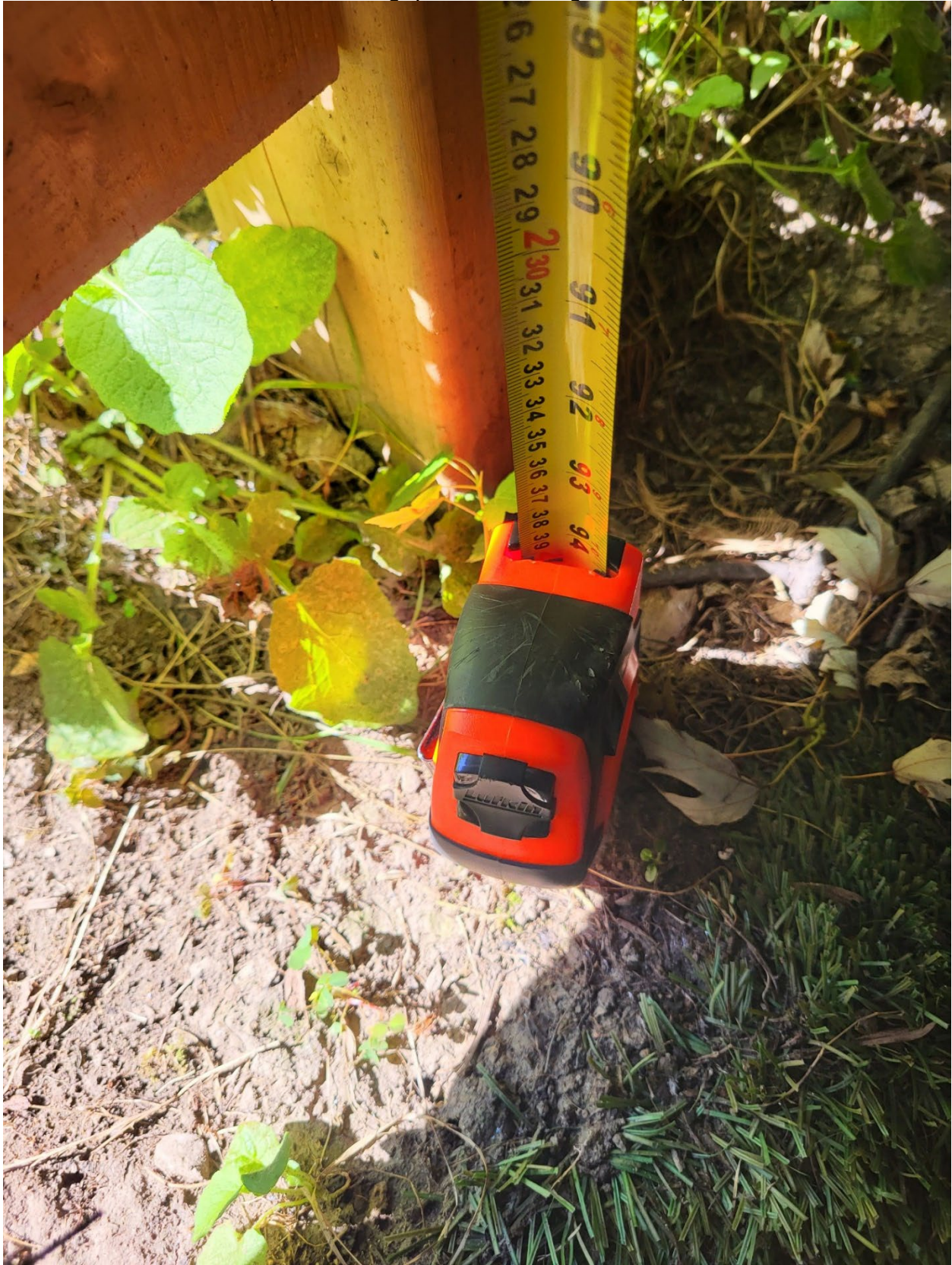
(West side gap under fencing 6 inches)
