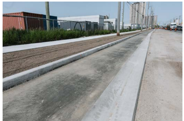
Figure 188. Cycle tracks under construction along Finch provide a curbed buffer between cycling infrastructure and the roadway (@FinchWestLRT on X.com)
