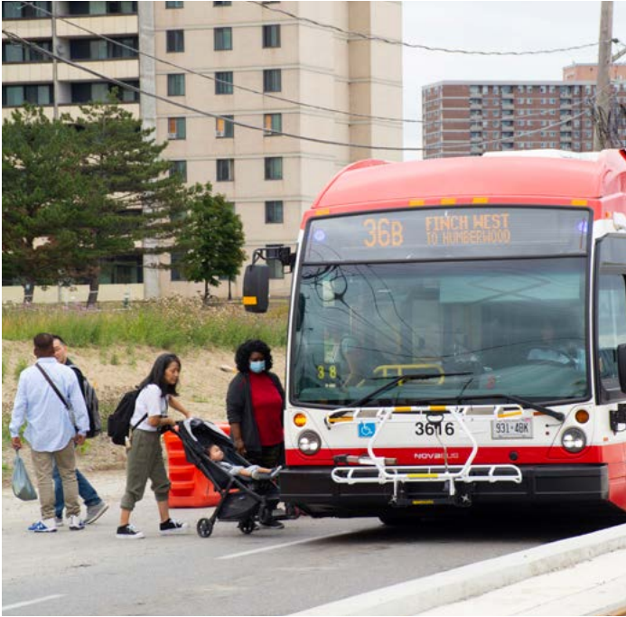
Figure 108. Passengers getting on the Finch West bus, in the midst of LRT construction (Perkins&Will)
