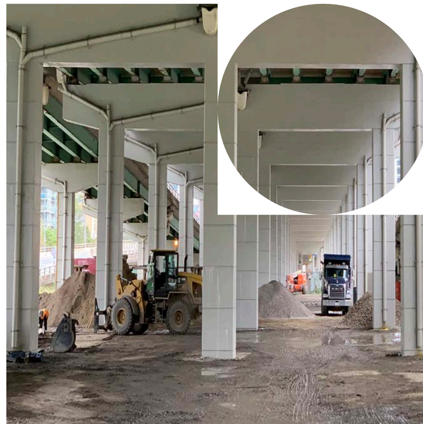
Image 37: View looking east of the Spadina Island site; note the construction materials and maintenance equipment.
