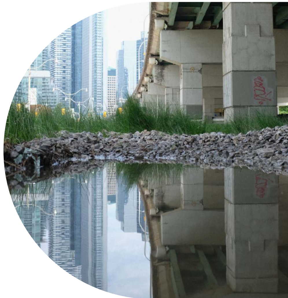
Image 21: View looking east toward Rees Street of pooling water and resilient plant life persisting along the edges of the elevated expressway.
