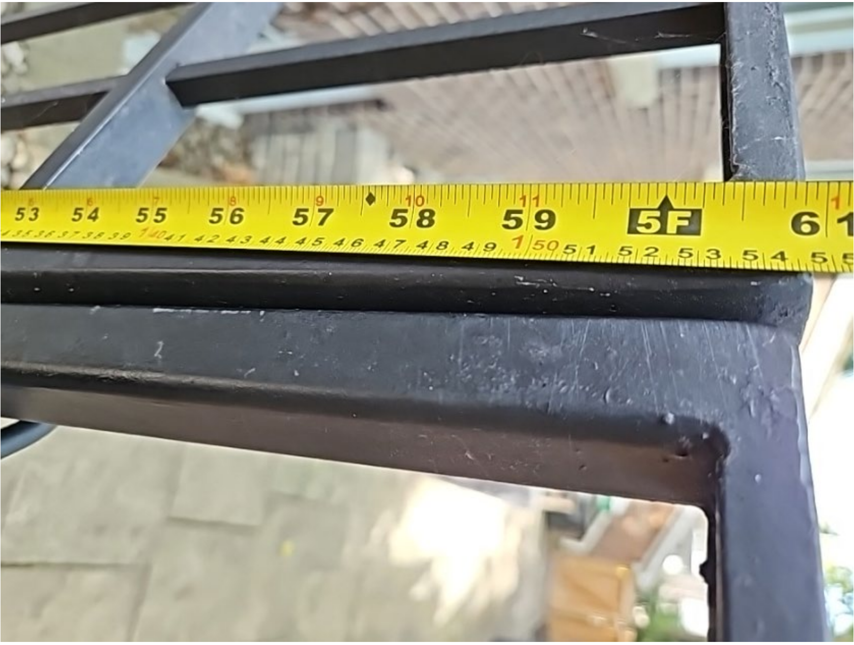
Attachment 4: Municipal Standards Officer's Photo - 19 Ivor Road - Existing Pool Gate Enclosure. — Rear Yard Gate
