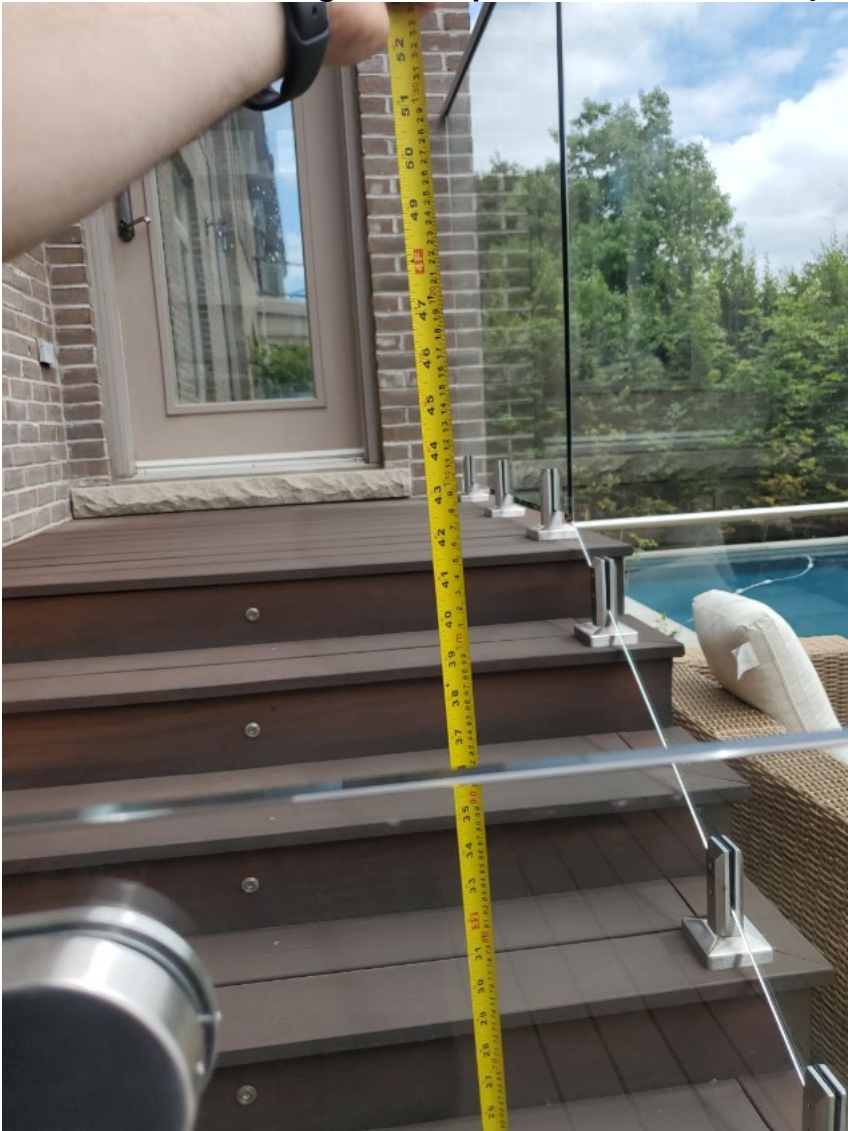
Attachment 4: The height of the pool enclosure from top of stair raiser.
