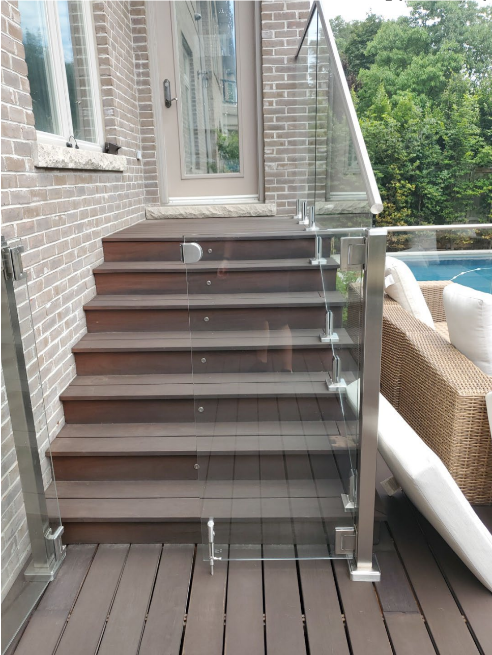
Attachment 3: The staircase from the deck forming part of the pool enclosure.
