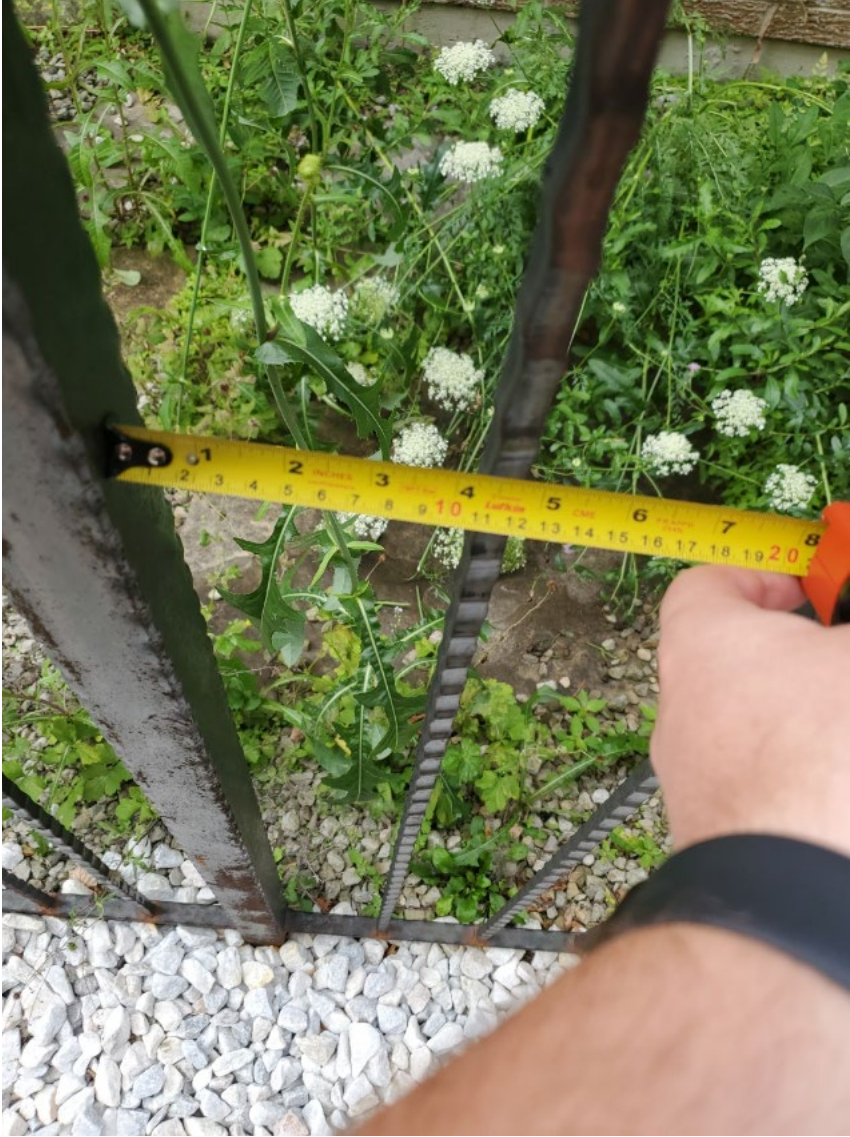
Attachment 2: Municipal Standards Officer's Photo 53 Yorkminster Road - West side of the existing pool enclosure.
